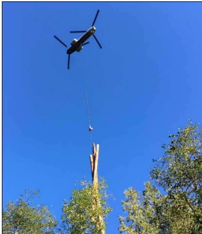
Figure 5-4 Example of LW being transported and placed with a twin rotor helicopter
