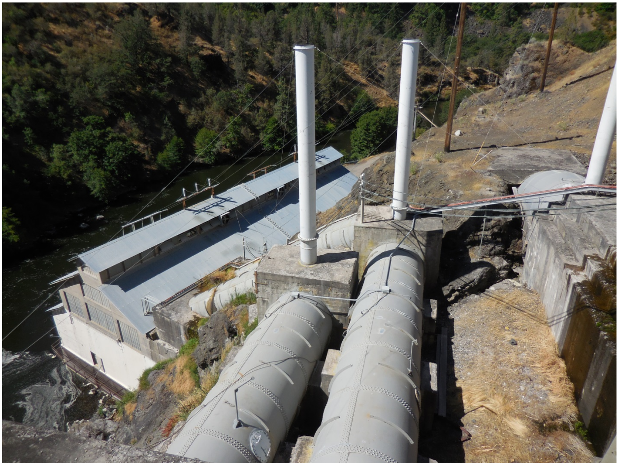
Figure 2.2-6 Copco No. 1 10-ft (left and middle) and 14-ft (right) Penstocks
