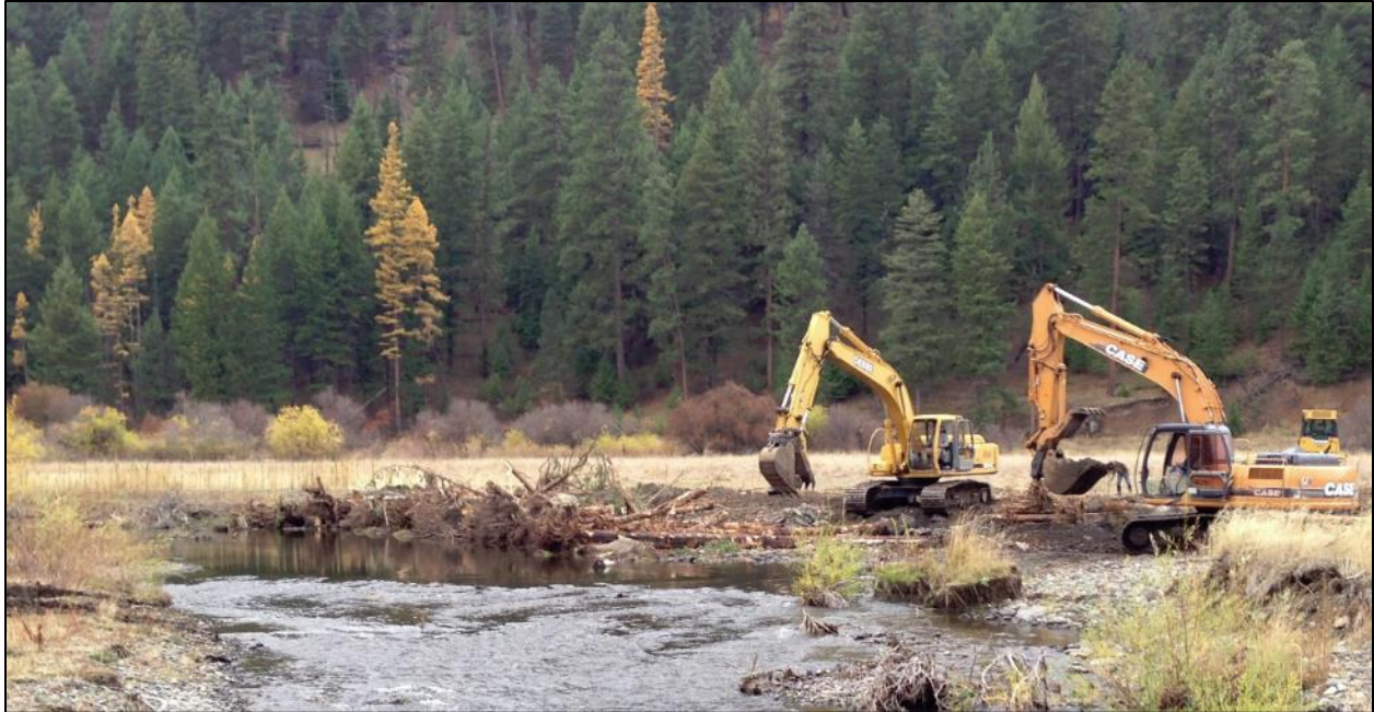
Figure 5-3 Example of LW structure being built for habitat benefits using ground-based equipment
