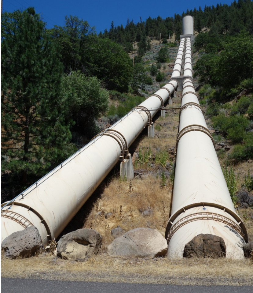
Figure 2.1-10 J.C. Boyle Penstocks
