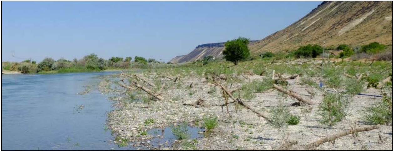
Figure 5-2 Example of restored floodplain area six months after construction showing new vegetation and wood roughness elements that provide habitat complexity and immediate, large scale roughness
