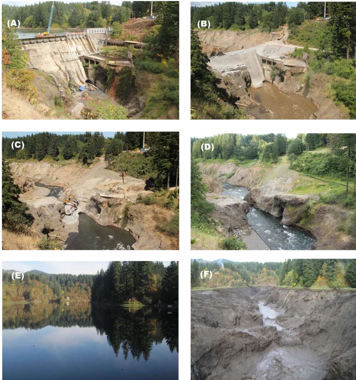
Figure 2. Decommissioning photos of Condit Dam as shown by photos taken by time-lapse cameras by Steve Stampfli of White Salmon, Washington. (A) The initiation of dam removal before the reservoir was drained, (B) approximately 75% decommissioned, (C) approximately 90% decommissioned, (D) 100% decommissioned. Photos (E) and (F) were taken by PacifiCorp staff on the day the reservoir was drained on 26 October 2011.
