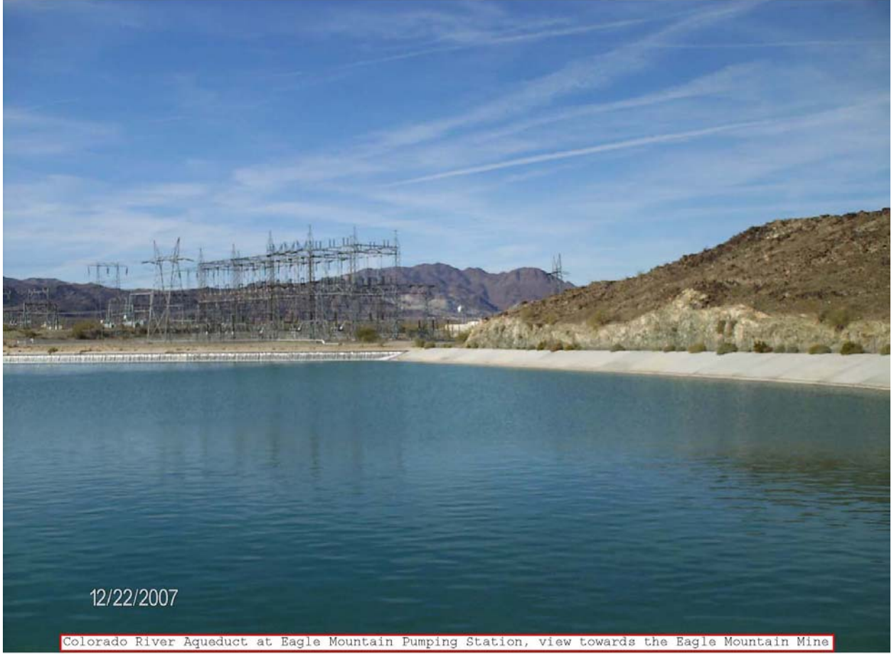
Photo 10. Photo of the Colorado River Aqueduct pumping station (2 of 2). Photo taken in 2007.
