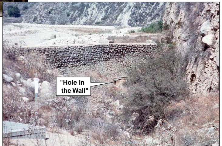
The "Hole in the Wall" in the Greenspot Bridge Retaining Wall
