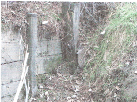
Remnant Pipe at Other End of Retaining Wall
