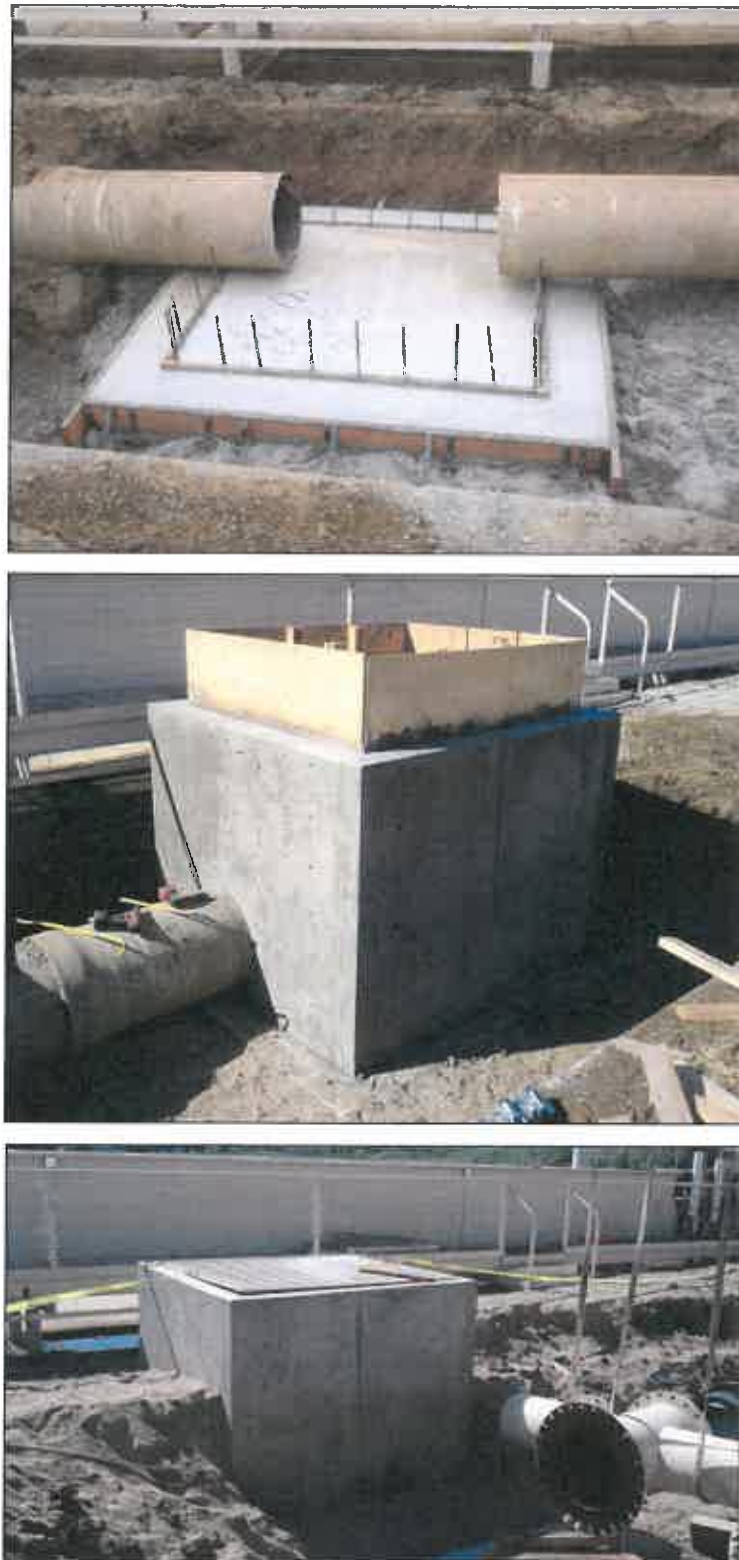
Figure A-2. Construction of the drain pipe connection box (right). Students in BRAE 433 (Fall Quarter) helped design and construct the bottom concrete slab shown in the top photo.
