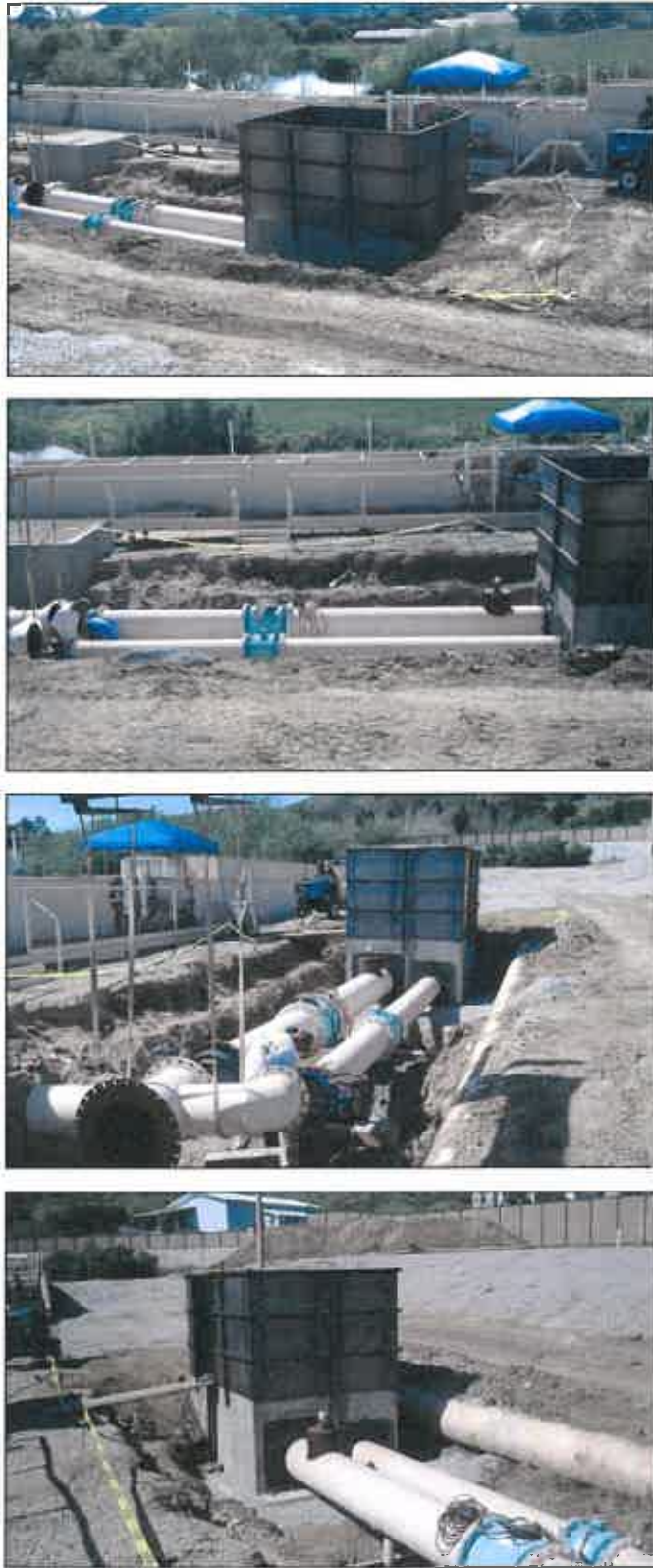
Figure A-4. Construction of the main spill box and 24” and 18” pipelines with magmeters
