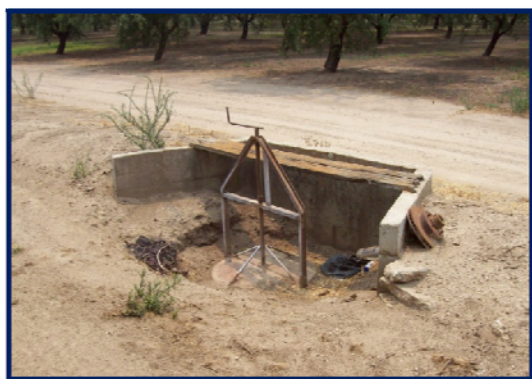
Figure 3-15. Orchard Valve Installed on SSJID Pipeline
