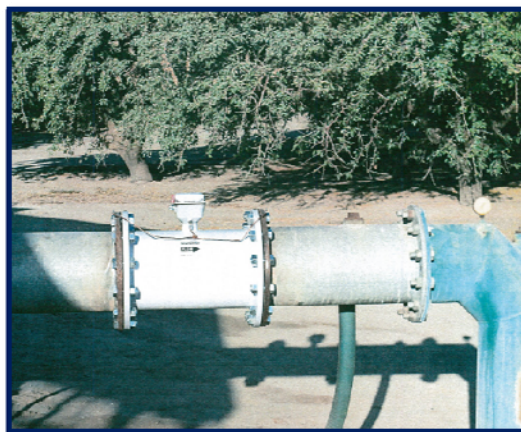
Figure 3-16. Magnetic Flow Meter
