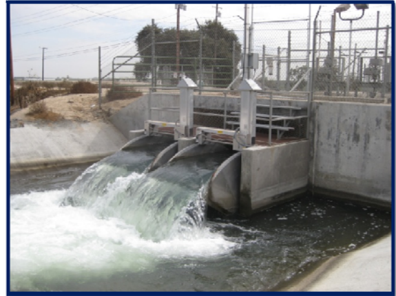
Figure 3-5. Flume Gates at Lateral Heading
