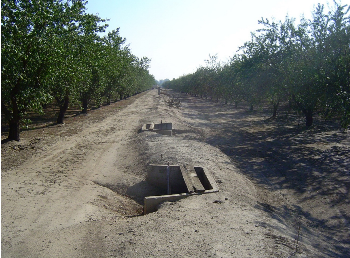
Figure A-2. Multiple valve turnout on a District pipeline.
