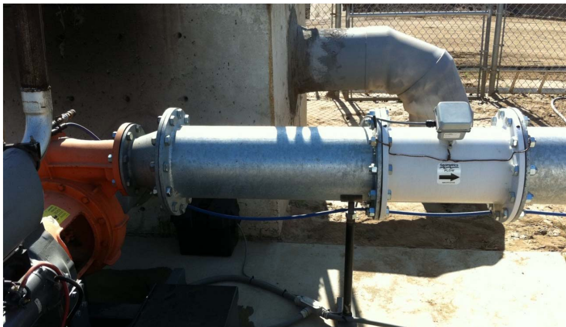
Figure A-5. Magnetic flow meter on delivery at Ra81.
