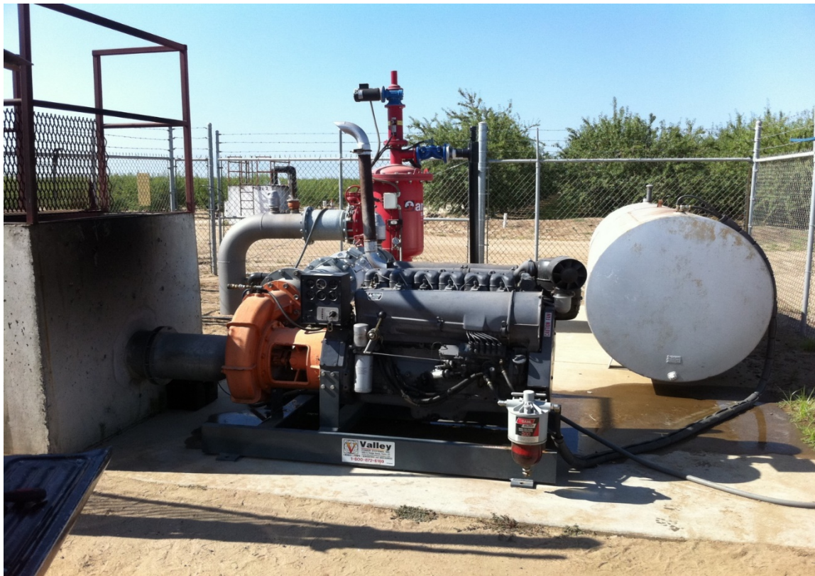
Figure A-1. Pump turnout on a District pipeline.
