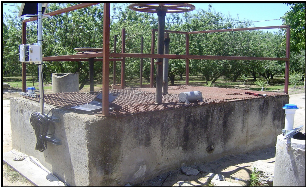
Figure A-3. Orifice gate turnout in a concrete box on a District pipeline.
