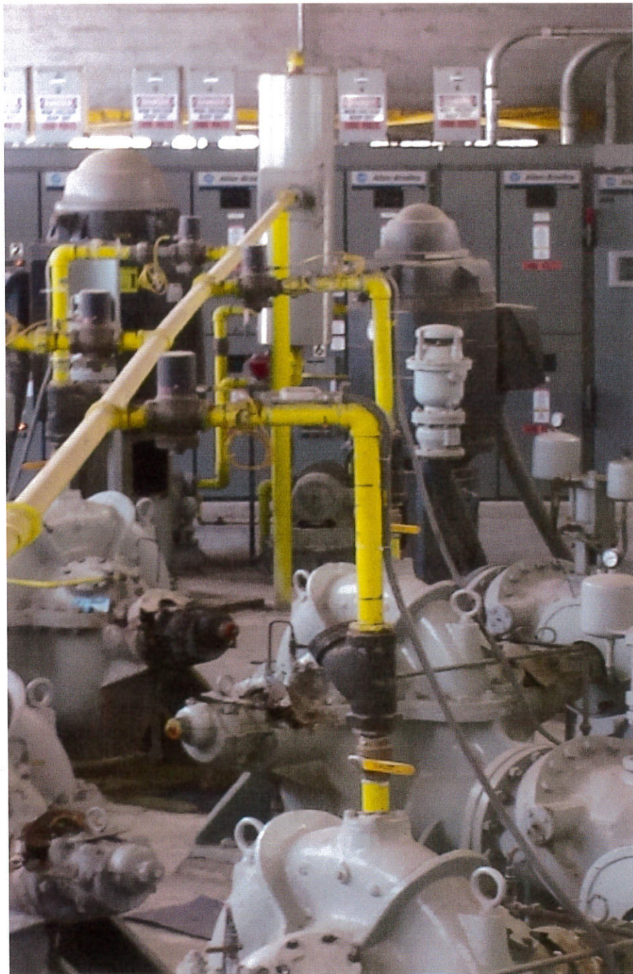
Photo 1: WSID Pump House. Gray pumps were turned off and the black pumps were running and capturing tailwater from Old River Cut.
