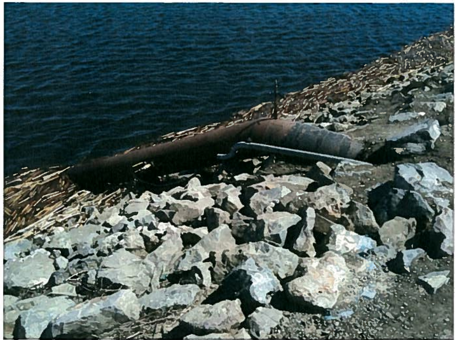
Figure 1: Velocity Sensor Installed on Water Side of Siphon
