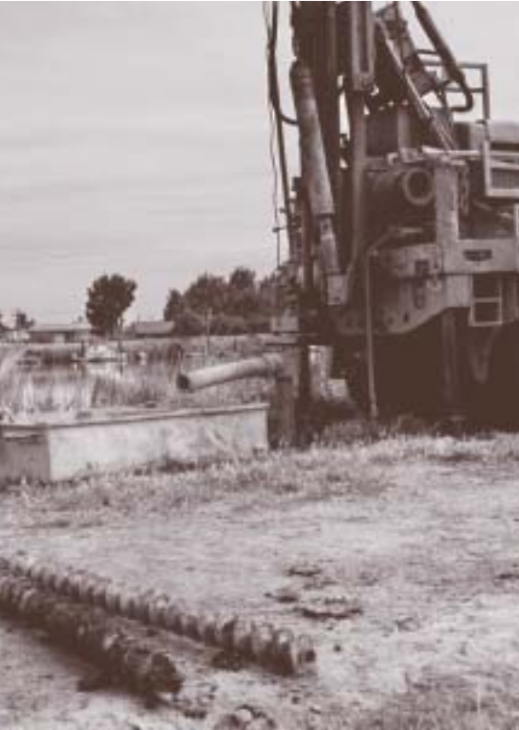
Core samples are taken on a Delta levee to determine the levee's integrity.
