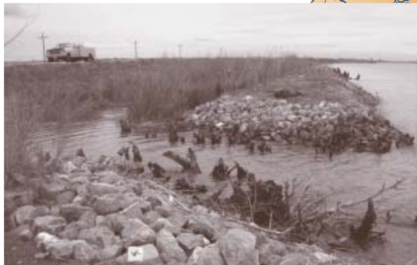
The Bay-Delta Levee System Integrity program funded special improvements projects like root wads used at the openings in the berm at the Twitchell Island setback levee to provide protection to small fish while stabilizing the embankment.
