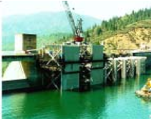
Installation of the Shasta Temperature Control Device took place between 1995 - 1997.
