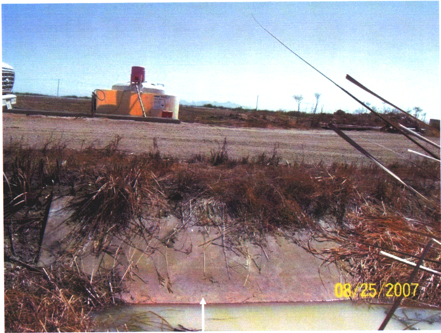
Effluent Receiving ditch, Point of Discharge is under water (Facing the East)
