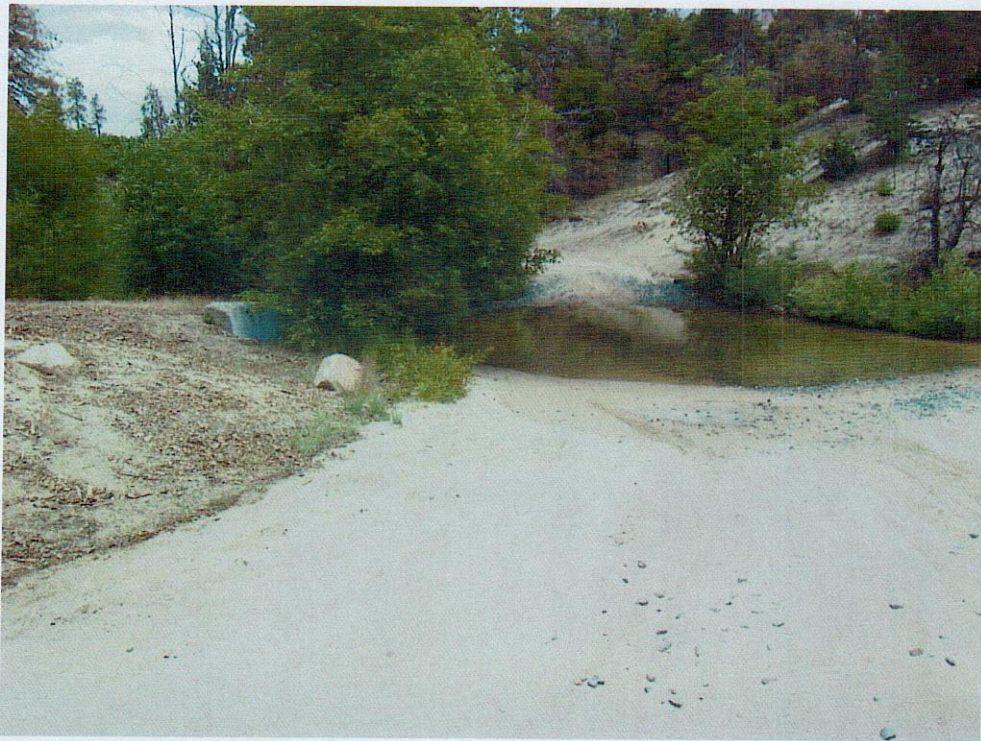
Less gravel seen - some likely buried. Road work removed rill entering the creek from the road. (June 2009, Robert Taylor)
