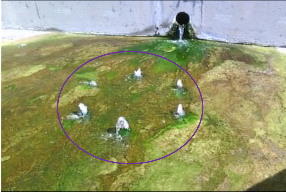
Figure 2. Manhole (Outlined by Purple Circle) Exuding Groundwater into San Jose Creek
