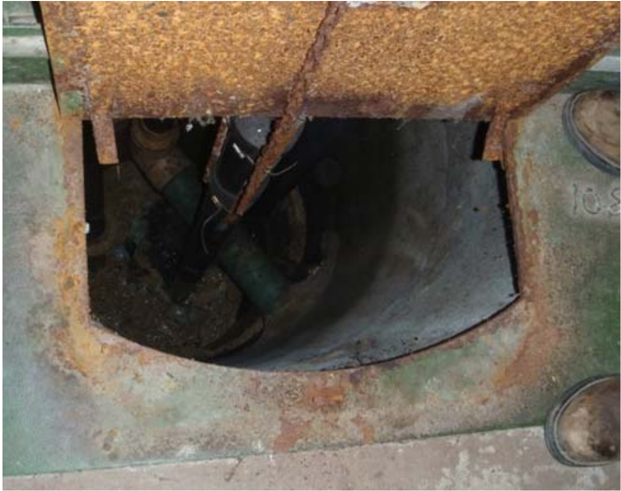
Photos 15: Orangewood lift station with significant corrosion and grease/solids in wet well
