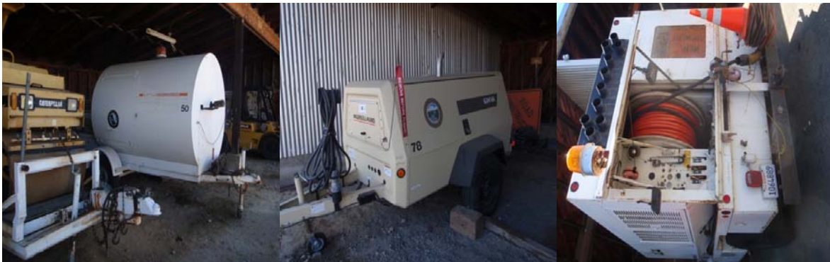
Photos 6-8: City maintenance shop [trailer mounted rodder (left), backup generator (center), and jetter (right)]
