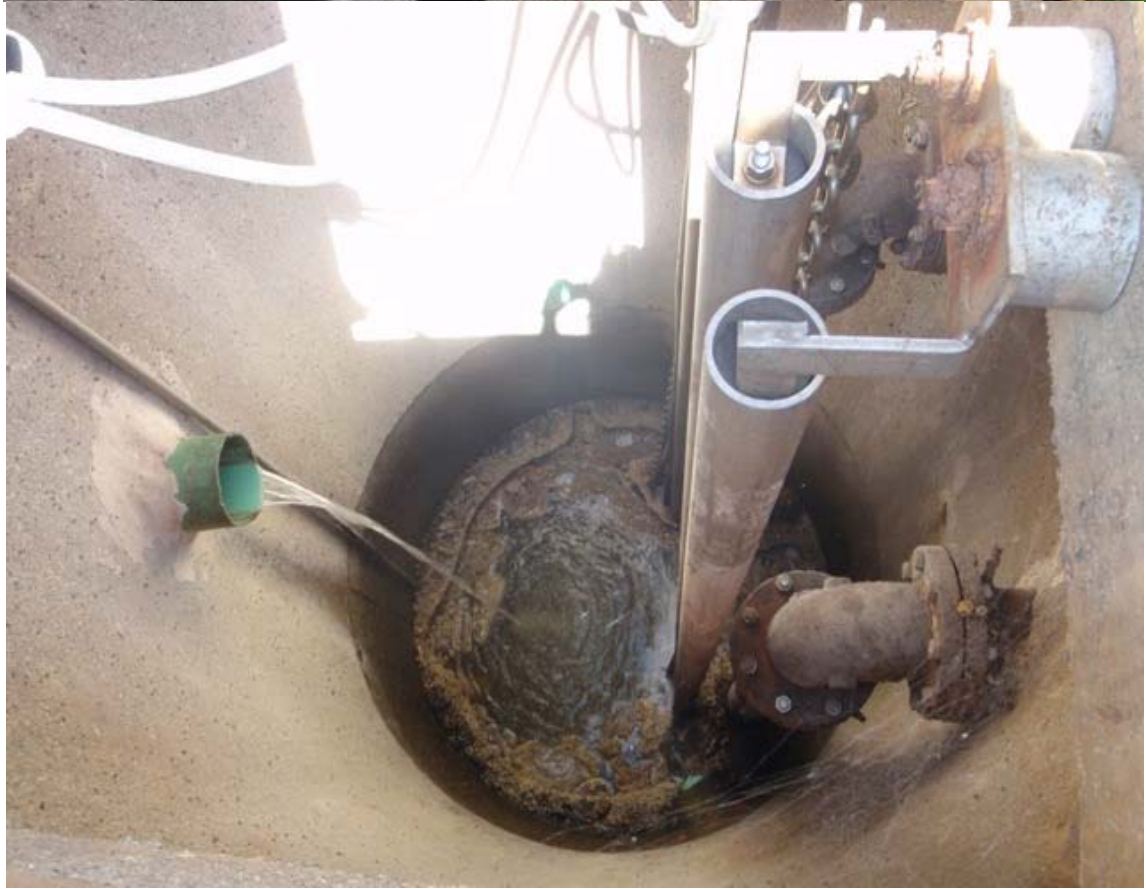
Photos 12-13: Riverview lift station wet well cover lifted (top) and wet well inside showing grease accumulation (bottom)
