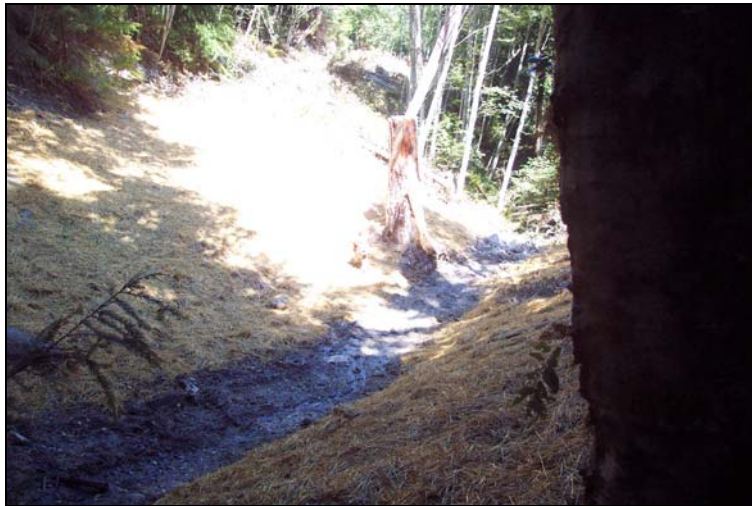
Site #8, the same stream crossing, post-treatment. The view is approximately the same as in the previous photo. Note the side slopes have been excavated back to the natural hillslope and mulched with straw. A tall stump approximately 18' high was unearthed during the excavation and is visible in the center of the photo.
