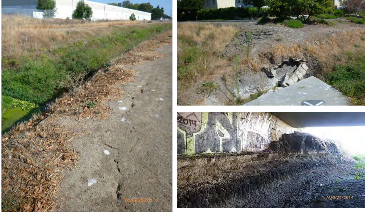
Left: Crack or fissures that indicate potential slumps. Note erosion control matting to left of crack. Top right: bank hardening that has become undermined by a lowering channel invert and high flows. Bottom right: Erosion beneath bridge piers.
