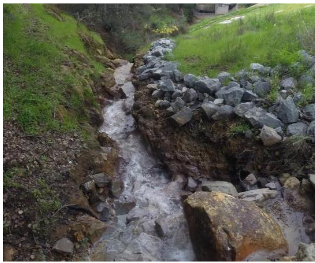
Figure 9. Same view after remediation.
