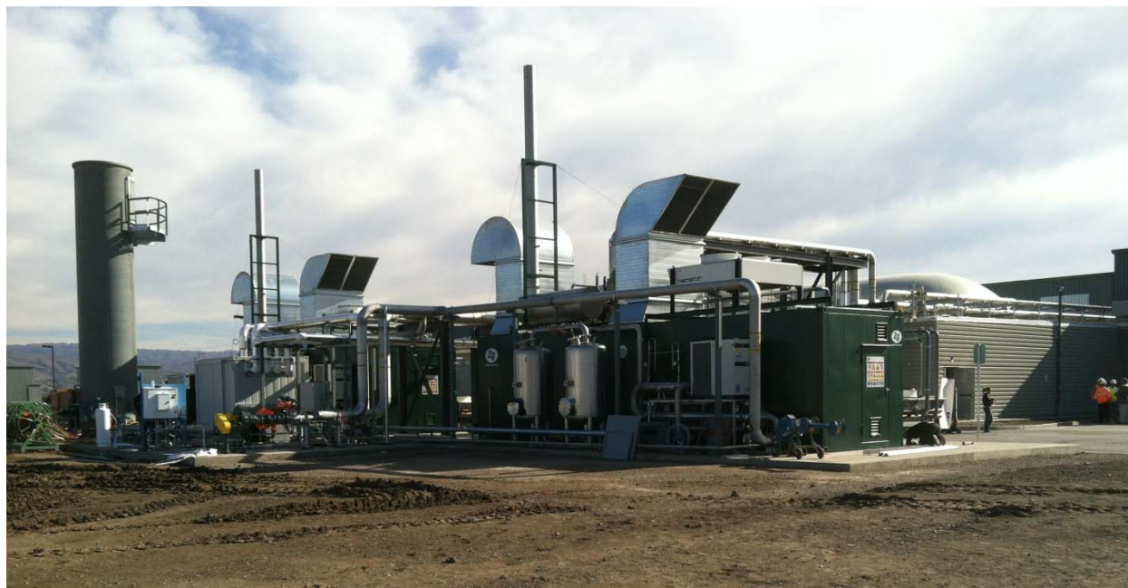
Photo 2. Anaerobic digestion facility in north San Jose.
