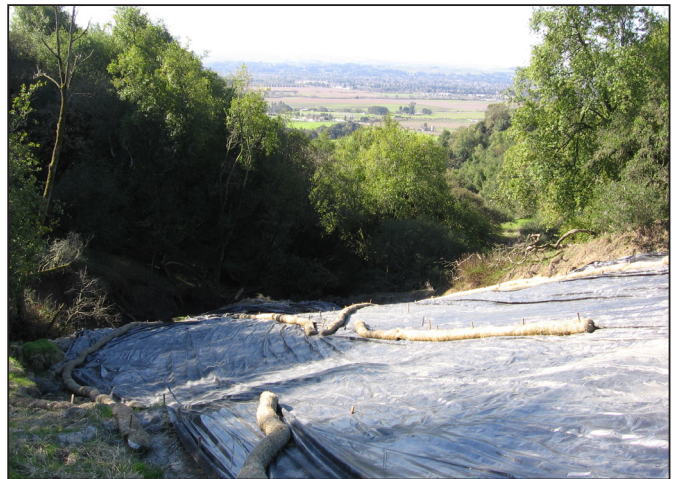
Photo d. Active lower slide face transports sediment directly to Cook Creek, this is below the area shown in Photo (c), plastics and wattles used to reduce slide saturation and erosion (Feb. 2006).
