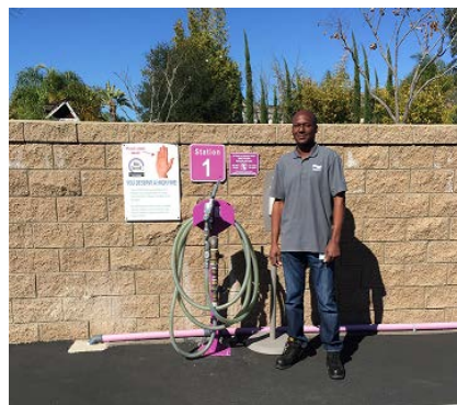
Dispenser at Fill Station
