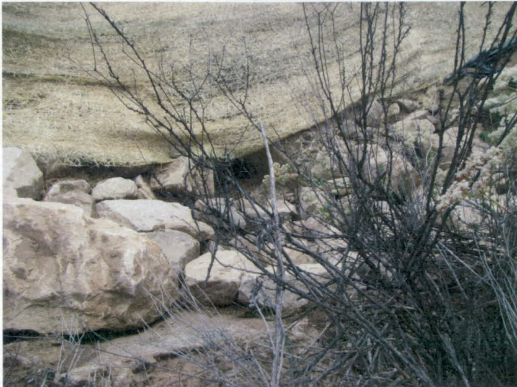
Photo 4: A second storm water inlet structure installed at the base of the fill at Drainage 2.
