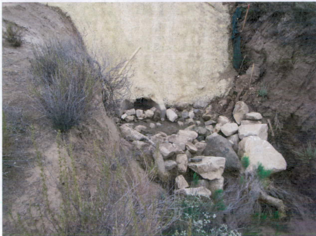
Photo 3: Storm water inlet structure installed at the base of the fill in Drainage 1.
