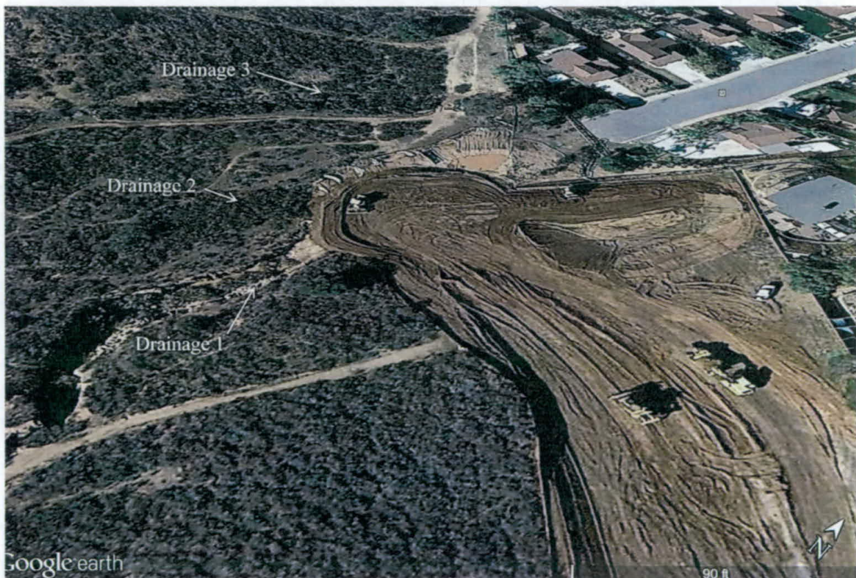
Figure 6. December 2014 Google Earth photo of initiation of grading activity for off-site road knuckle.
