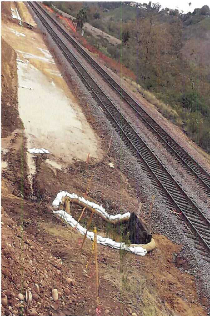
Photo 15 shows discharge point #3 due to inadequate sediment and erosion control (shown in Photo 7).
