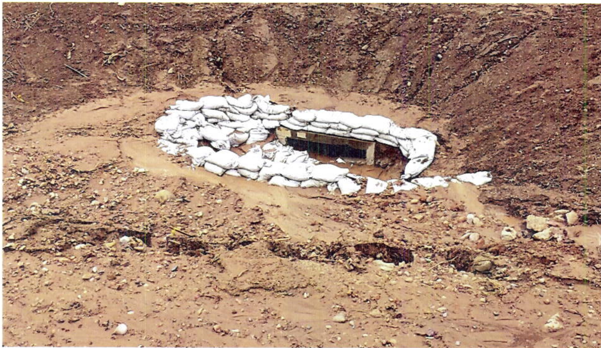
Photo 12 shows discharge from easternmost "bowl" due to inadequate perimeter, sediment, erosion, and runoff controls.
