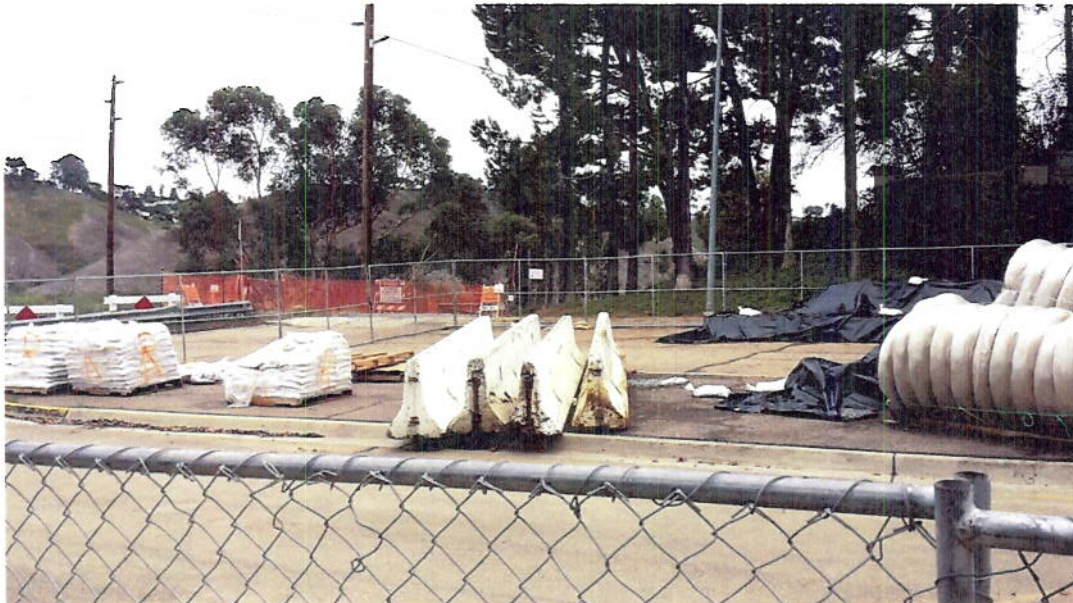
Photo 16 shows additional BMPs (gravel bags and wattles) on site, but not in use.
