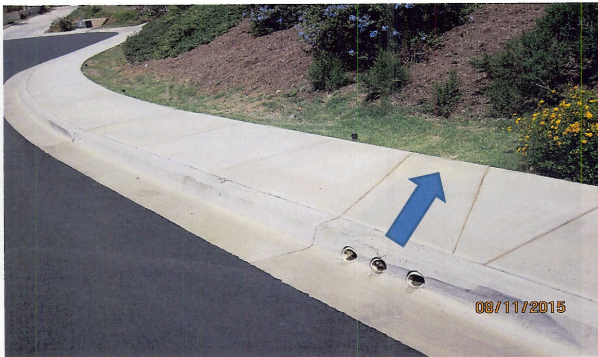
Photo 3(h): Inlet pipes upgradient of swale are buried beneath turf rendering the inlet structure to the swale inoperable.
