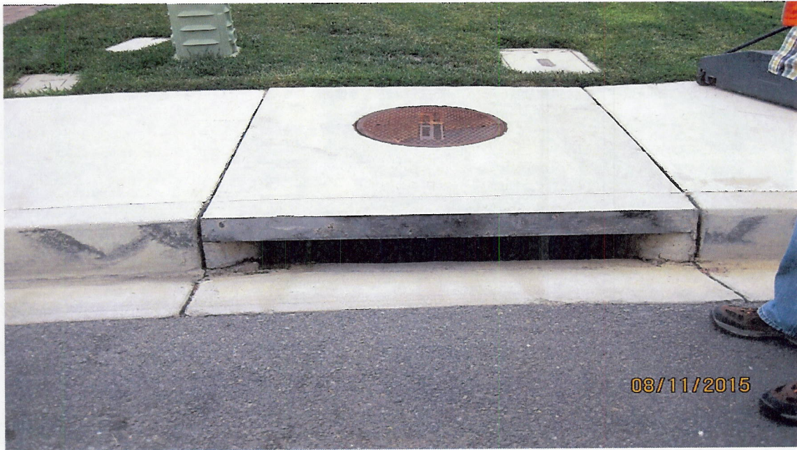
Photo 2(b): Single drainage inlet at end of Trovita Court. Inlet picks up flow from entire subdivision. According to the City there is a low flow inlet and high flow bypass associated with the inlet.
