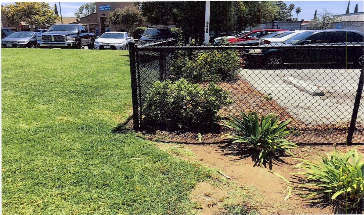
Photo 4(c): Second bioswale should be in line with white post, but area lacks vegetation and is not contoured as a swale. Missing BMP.
