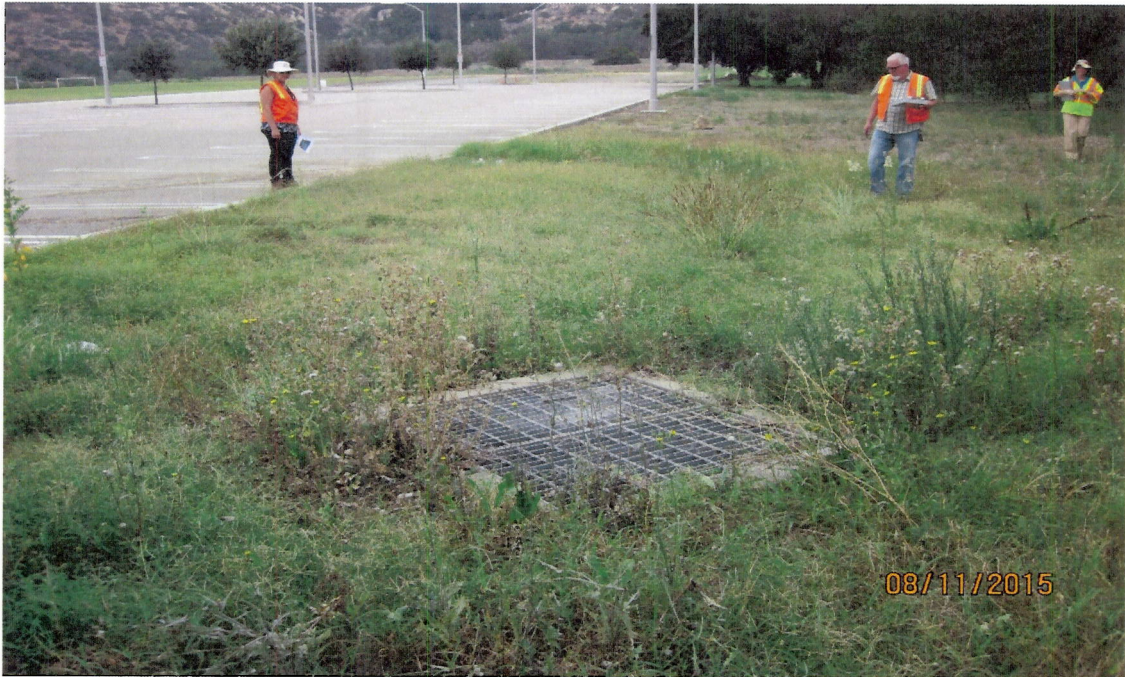
Photo 1(c): Bioswale is fully vegetated, but flow path tends to be slightly uphill from inlet to outlet. Entire area may function to allow infiltration of runoff. But re-contouring necessary to allow bioswale to perform as designed. City should inform Public Works Dept. that swale is in need of maintenance.
