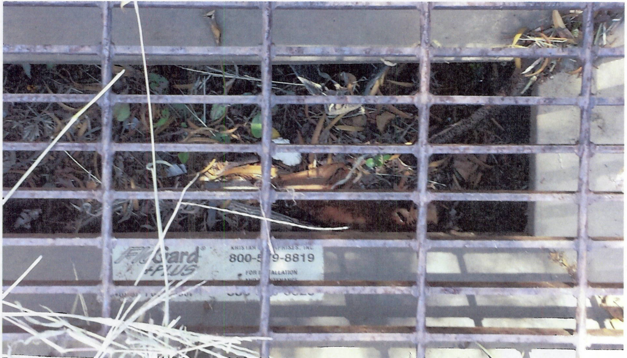
Photo 4(d): Inlet filter in place on street outside of property, and in need of maintenance.
