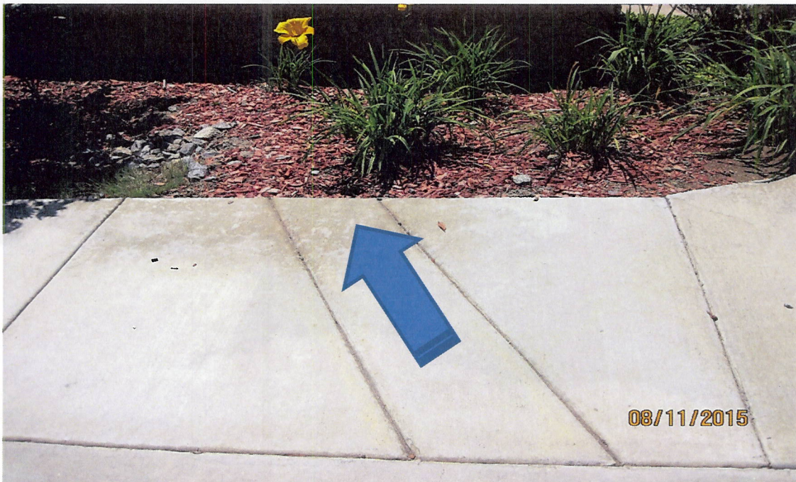
Photo 3(g): Inlet pipes upgradient of swale are buried beneath ornamental landscaping rendering the inlet structure to the swale inoperable.
