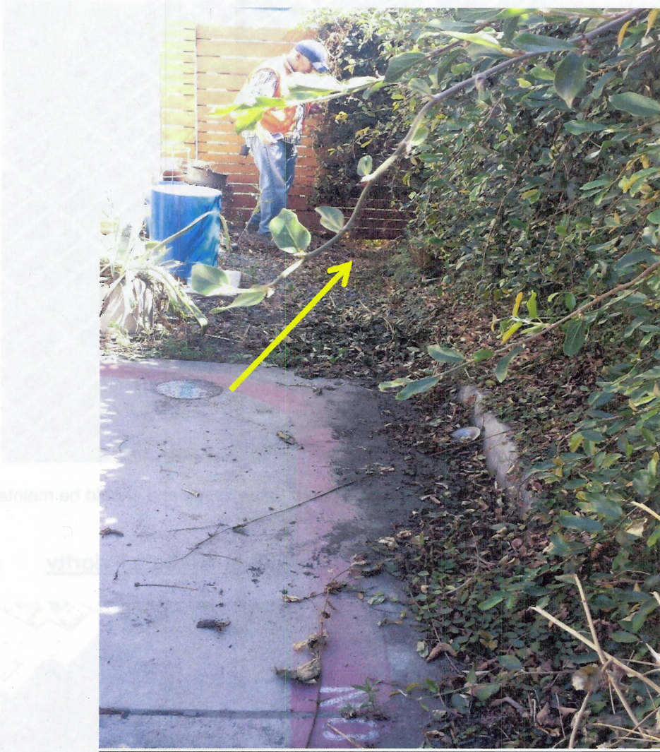
Photo 7(b): End of impervious surface in the interior of the apartment complex. Sediment build up is apparent. Arrow shows the inlet to the bioswale under the fence of a resident's private side yard.
