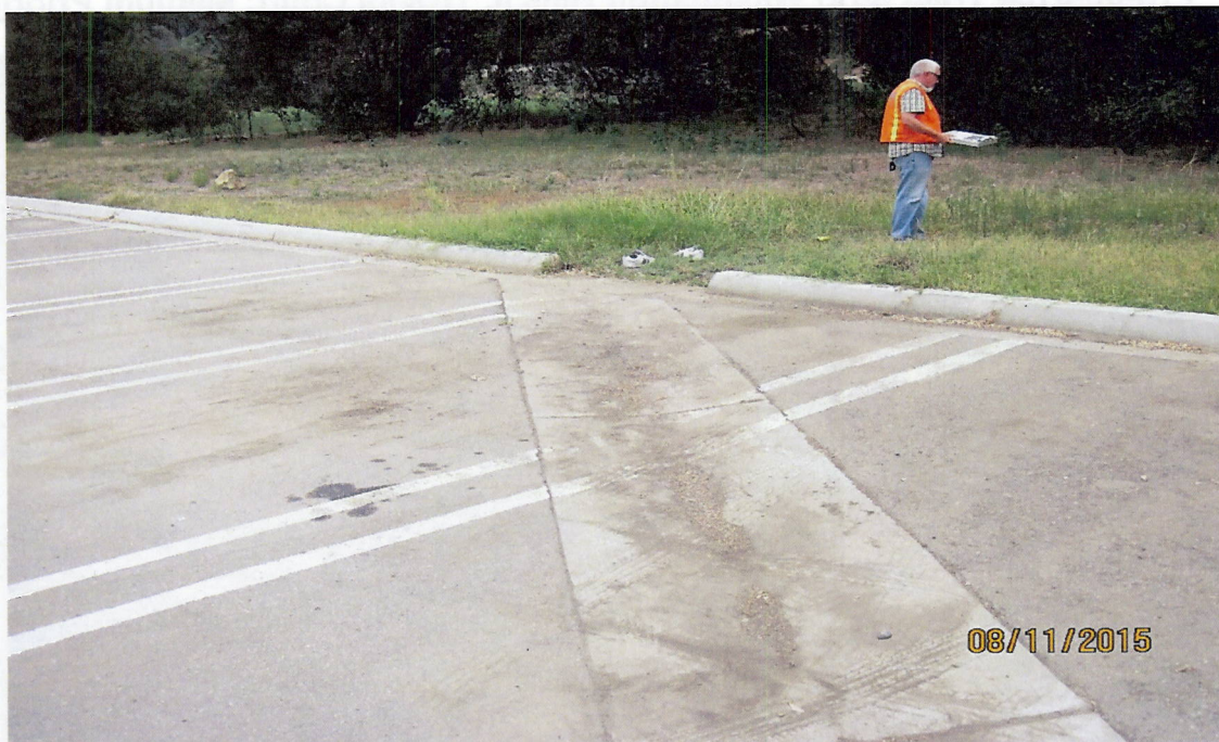
Photo 1(b): Inlet to bioswale from parking lot, ground higher than inlet preventing flow to enter swale, trash present, needs maintenance and contouring to allow flow to enter swale. Evidence of sediment buildup at inlet. Parking lot could use a sweeping.
