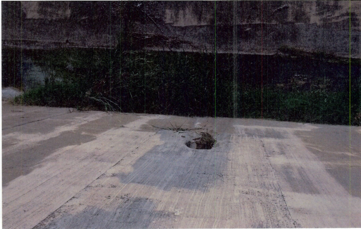
Photo 2(f): Hi flow outlet to Escondido Creek showed signs of moisture at terminus. Potential bypass of low flow outlet to swale.
