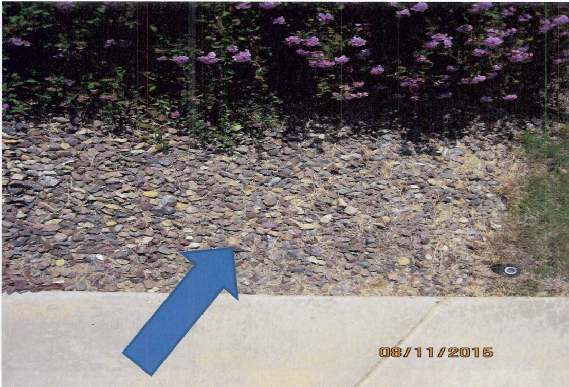
Photo 3(f): Inlet pipes upgradient of swale are buried beneath hard packed dirt and gravel rendering the inlet structure to the swale inoperable.
