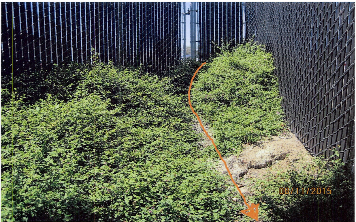
Photo 6(d): Bioswale is situated on steep slope with no vegetation in the flow path. Poor design.
