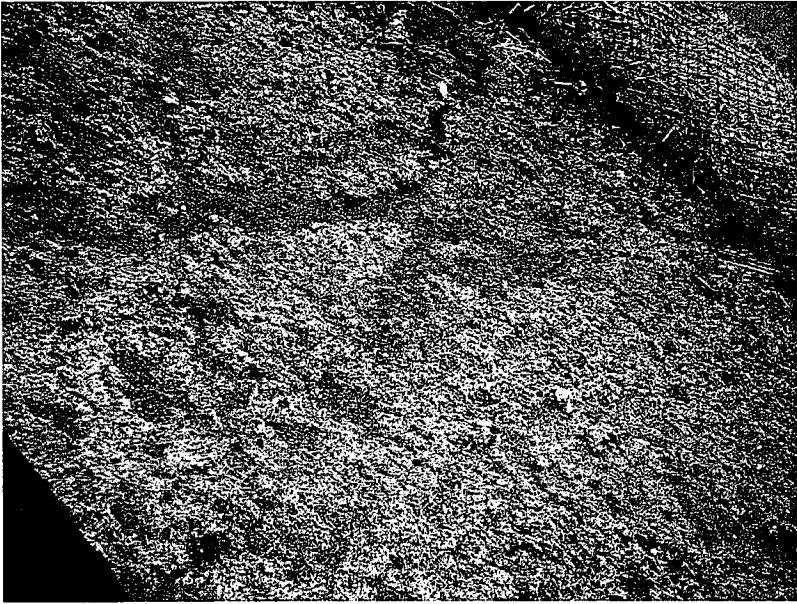
712. A closer look at the erosion control on the banks shows the inconsistent application.
