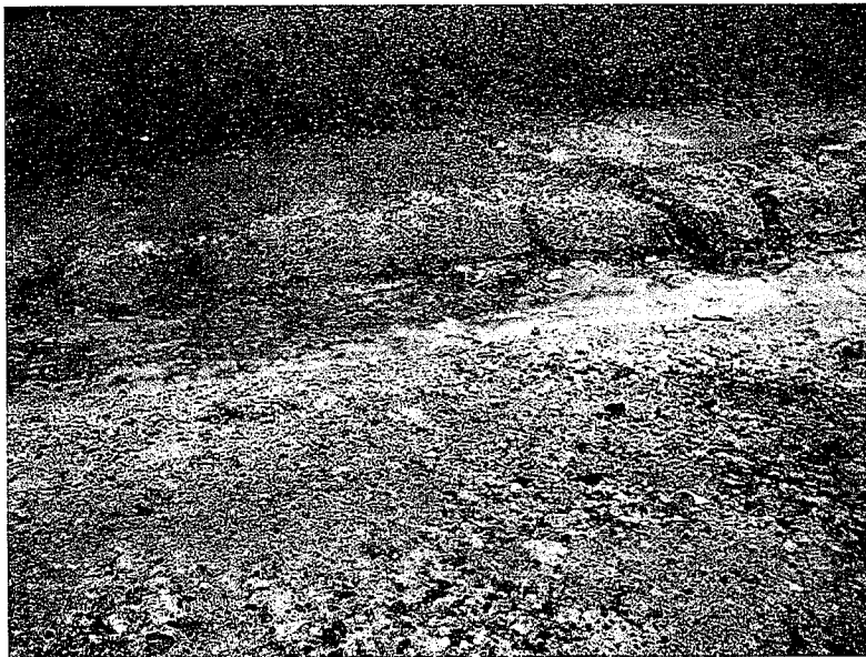
690. The storm water in the channel is clear on the left of the photo and then picks up sediment as it flows to the right in the unlined dirt channel.
