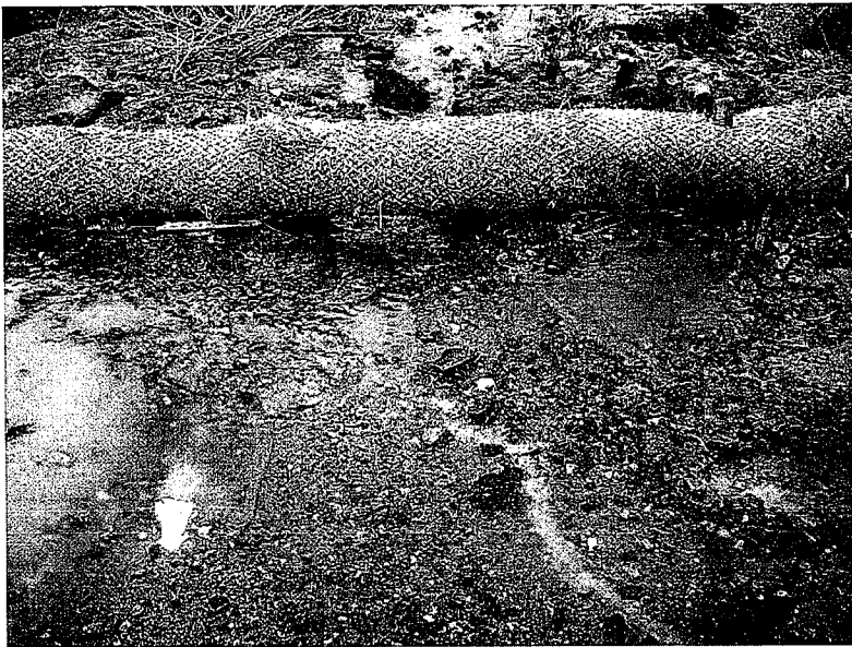
697. Sediment laden water from the construction site is running under the fiber roll in photo 695 and discharging into Loma Alta Creek.
