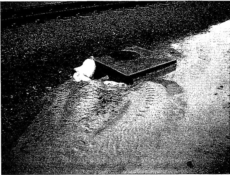
685. A closer look at the storm drain inlet in photo 684.
