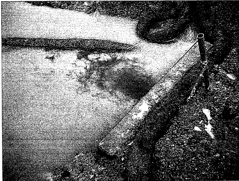
679. This is the inlet receiving the sediment laden water in photo 678. The inlet has backed up and clear water was bubbling out.
