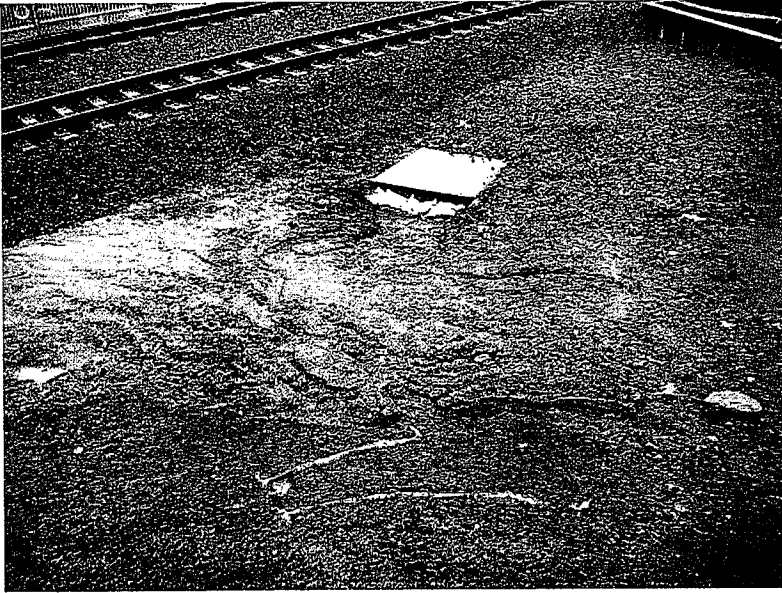
727. Storm drain inlet is blocked off with gravel bags. No ponding water suggests that storm water flowed elsewhere.
