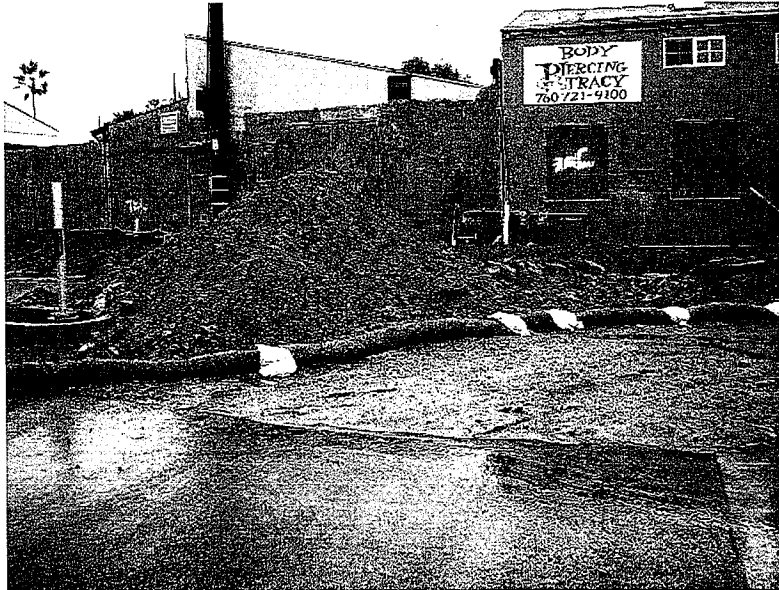
683. Stockpile has a fiber roll around it. Construction exit does not have BMPs to prevent sediment tracking. These deficiencies were also noted on Tuesday, November 27, 2007. Sediment on the pavement has since been swept up.
