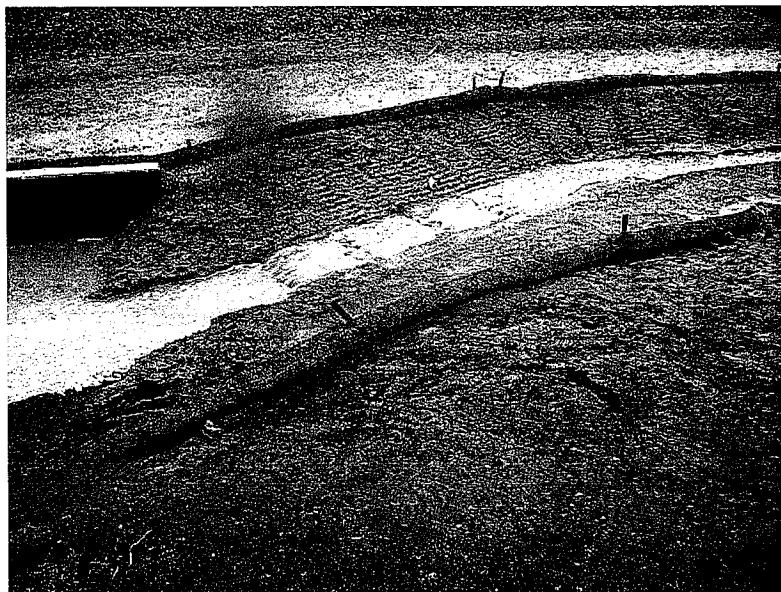
673. The bed of the unlined dirt channel is eroding away.
