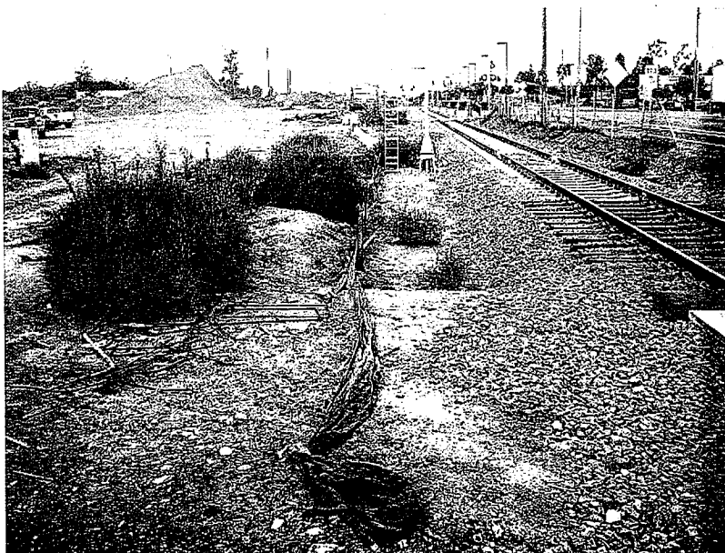
12. Silt fencing has not been maintained along the south side of the tracks. Photo looking west.
