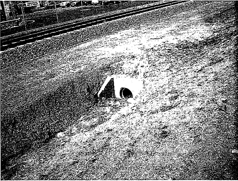
4. Another storm drain inlet along the north side of the tracks is without sediment controls such as gravel bags. Trash in the drainage ditch. Photo looking west.
