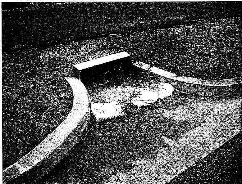
8. Storm drain inlet along the south side of Washington Avenue has BMPs that have not been maintained. Photo looking south.
