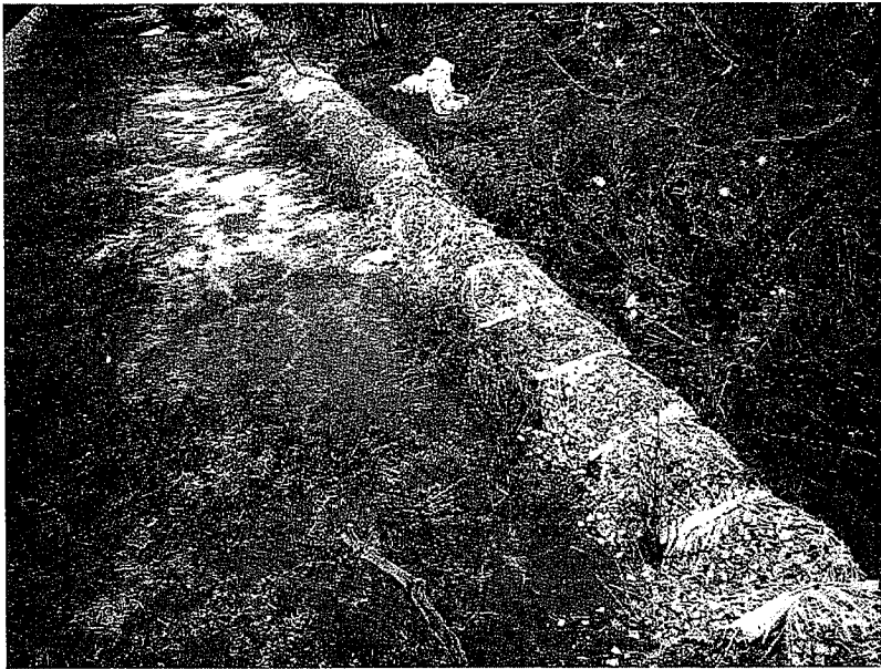
20. Gravel bags along north Barham Drive have not been maintained. Photo looking north.
