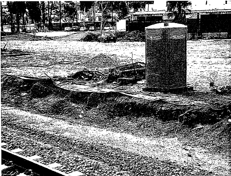
14. Silt fence is unmaintained. Construction debris and trash is not protected from storm water. Photo looking south.
