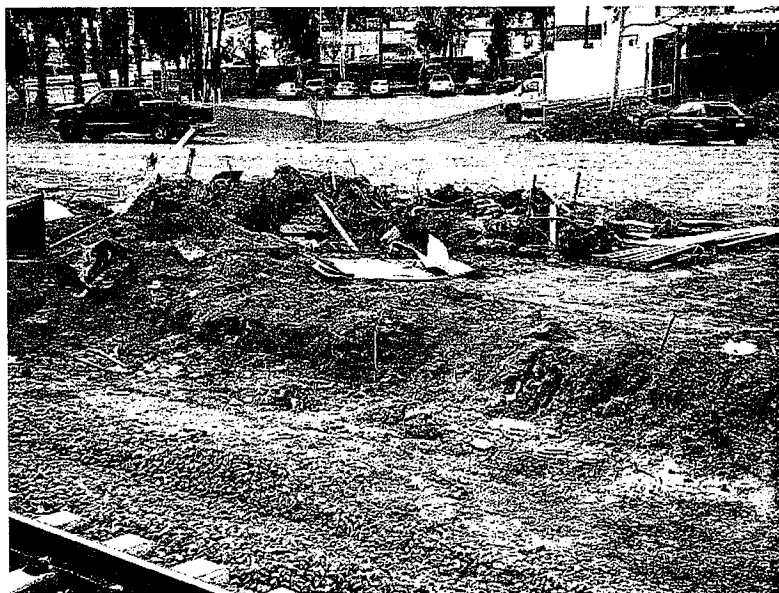
15. No silt fence is implemented in this area. Construction debris and trash is not protected from storm water. Photo looking south.
