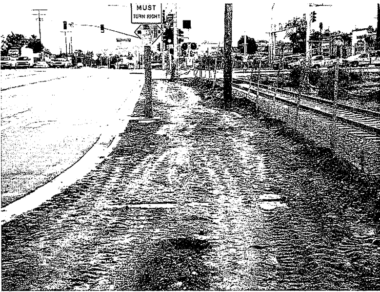
16. Bare soil north of the tracks does not have sediment controls or soil stabilization. Photo looking east.
