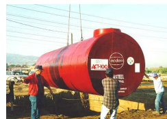
Underground storage tank
