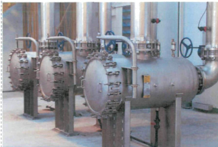
Sweetwater Authority's demineralization facility
