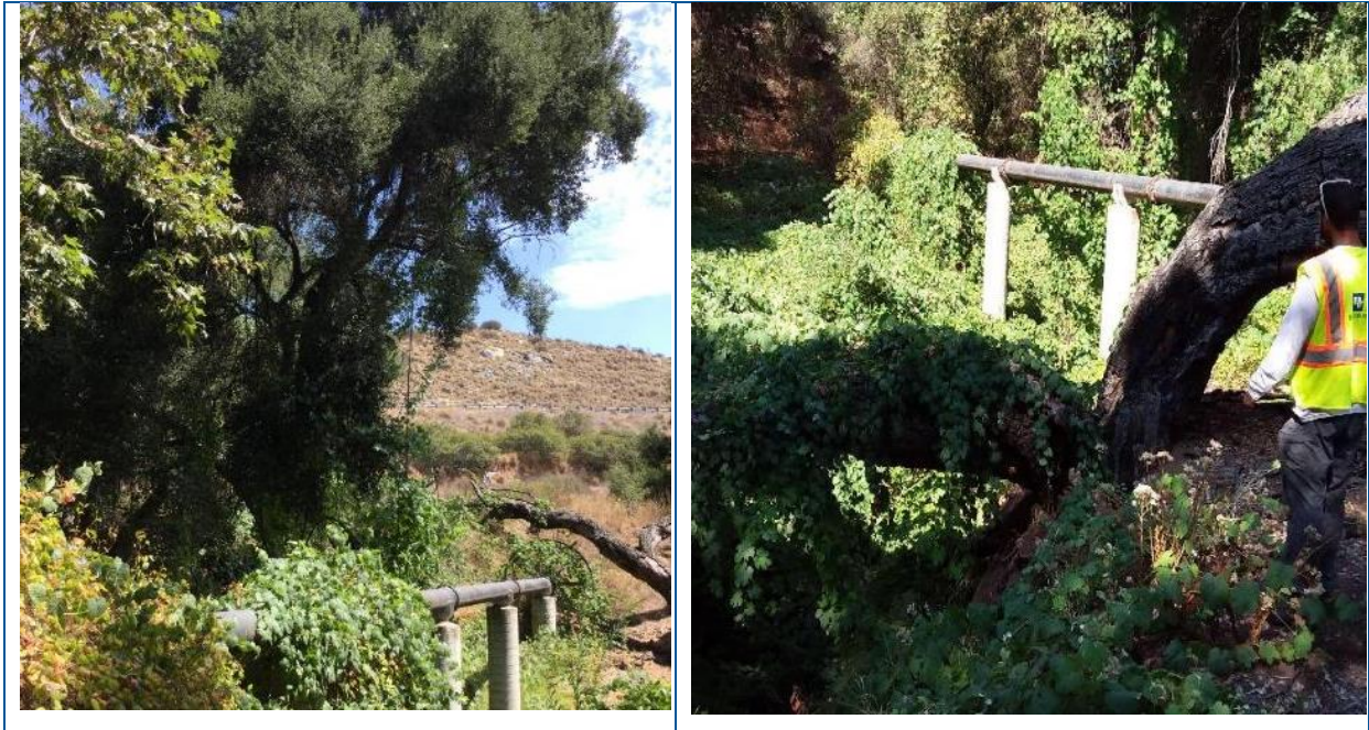
Figure 12 Examples of trees leaning into a stream because of stream bank erosion
