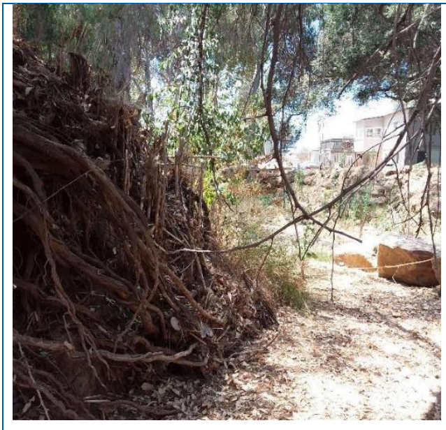
Figure 11 Example of excessive root exposure due to stream bank erosion
