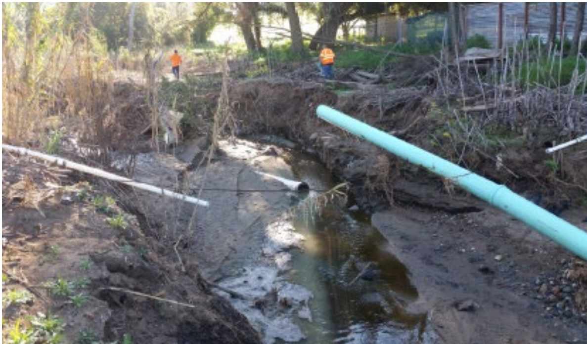
PHOTO 1: Damaged 12-inch PVC sewer line in Los Coches Creek. (photo by SD Sanitation District)
