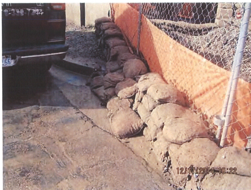
Photo 1. Evidence of sediment discharge at Akins entrance/exit
