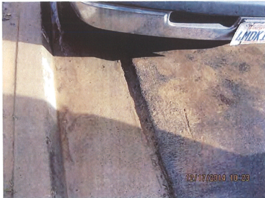
Photo 3. Sediment accumulation along Akins curb gutter, downstream of Akins entrance/exit
