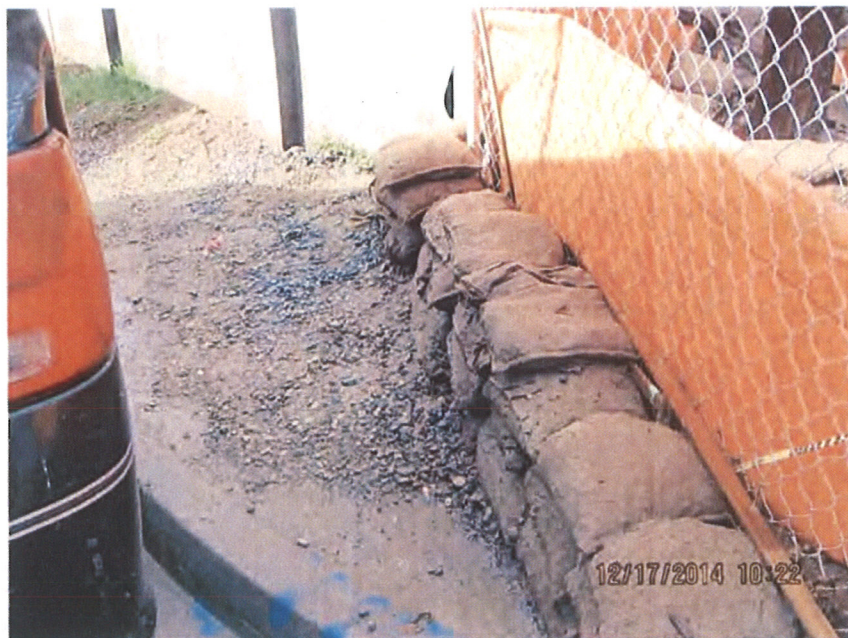
Photo 2. Evidence of sediment discharge at Akins entrance/exit
