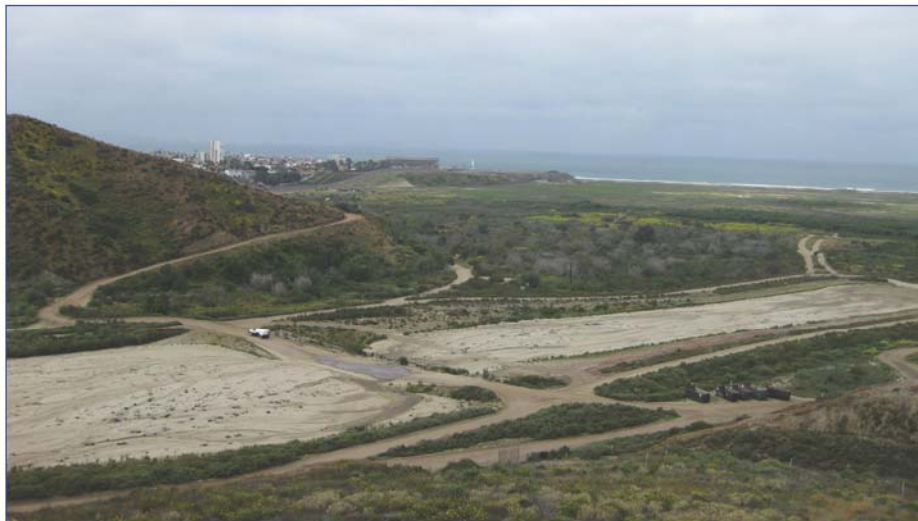
Sediment basins constructed in the Goat Canyon can capture up to 60,000 cy of sediment in wet weather flows.
