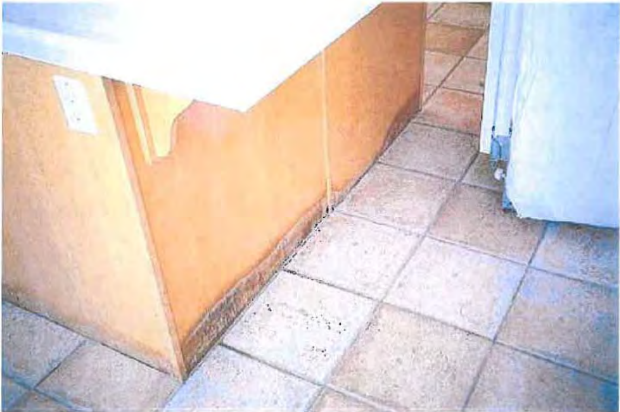
Photo 4- water migration through slab into cabinetry
