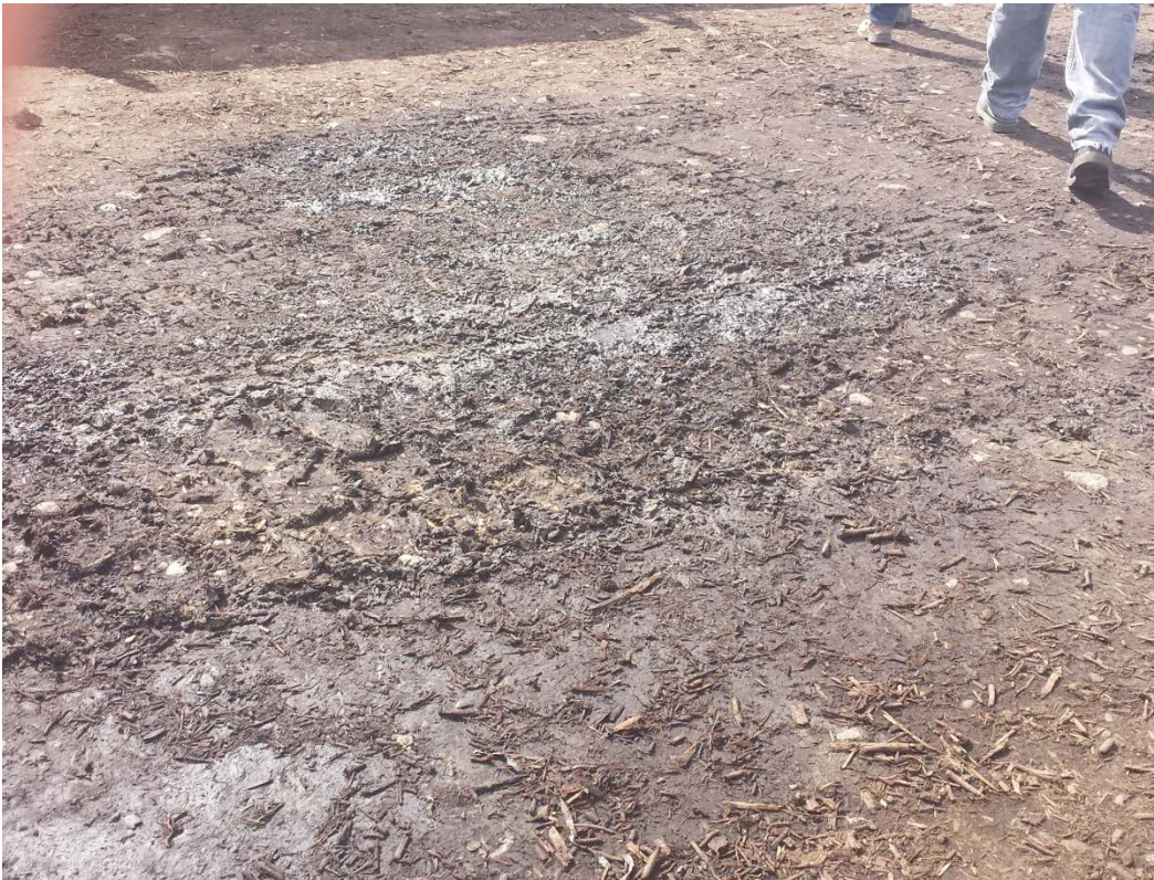
Figure 4: Photo of overwatering from dust control truck.
