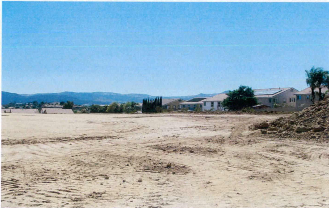
Photo 6: Upper proposed residential pad is inactive, and devoid of erosion control BMPs in violation of Order 2009-0009-DWQ and 401 certification conditions.
