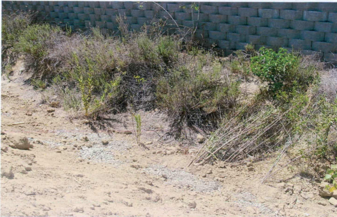
Photo 3: Stockpile removal and grading activities have resulted in sediment discharge into mitigation area and impacts to native vegetation (mulefat plantings are knocked over by sediment in this photo). These discharges of sediment are in violation of discharge prohibitions in the Basin Plan For the San Diego Region, Order 2009-0009-DWQ and 401 cert 08C-073. Photo taken 07/03/14.
