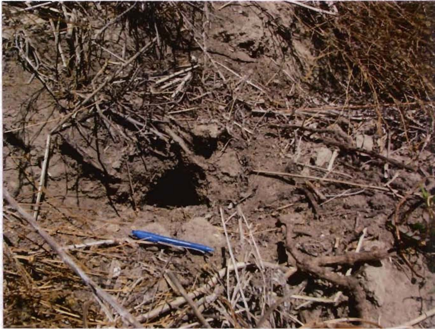
Rodent holes and mounds in the cover in the southeastern quadrant of the Landfill near Pacific Street.
