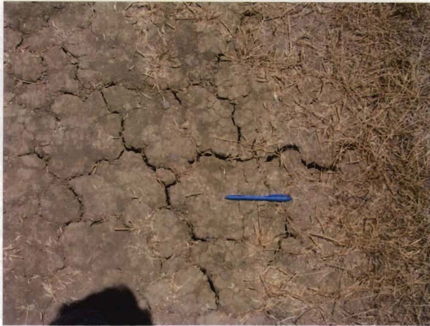
Cracks in perimeter road in the southeastern quadrant of the Landfill.
