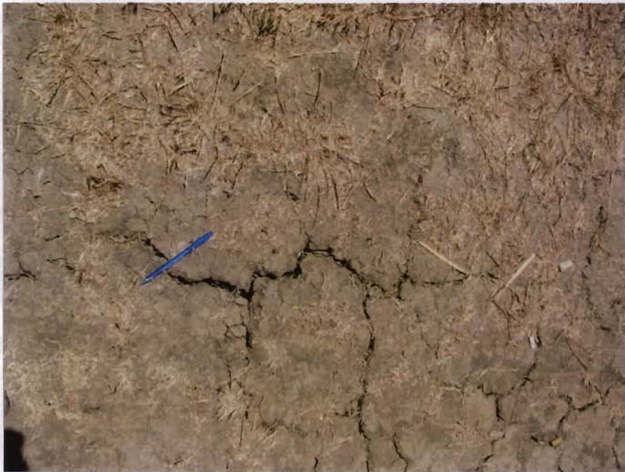
Cracks in the perimeter road in the southeastern quadrant of the Landfill.
