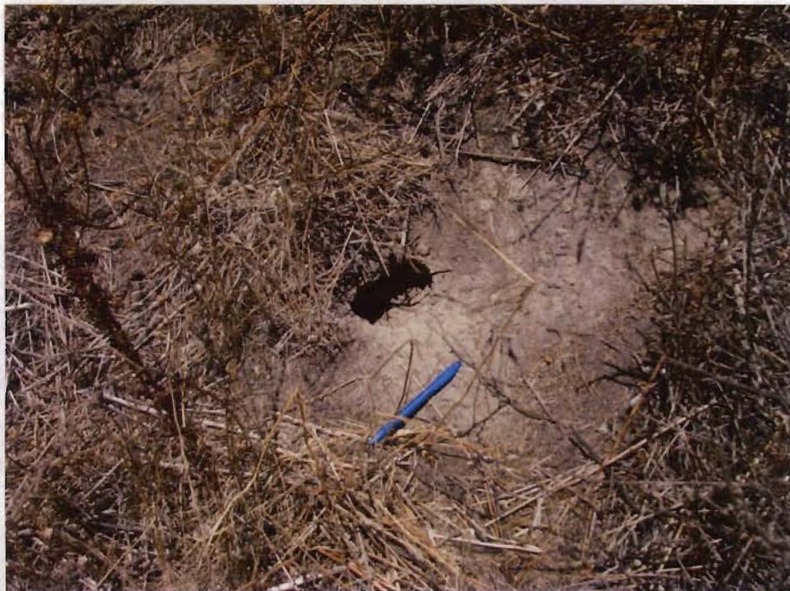
Rodent holes and mounds in the cover in the southeastern quadrant of the Landfill near Pacific Street.
