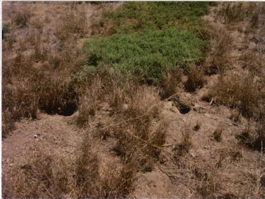
Rodent holes and mounds in the cover in the southeastern quadrant of the Landfill near Pacific Street.
