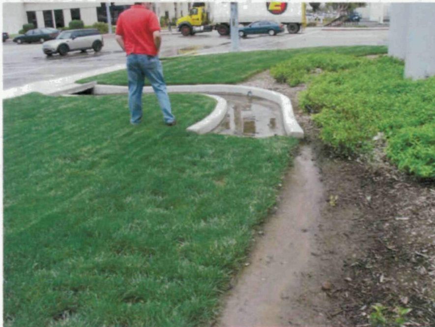
Figure 14. Outlet for Bioswale 2
