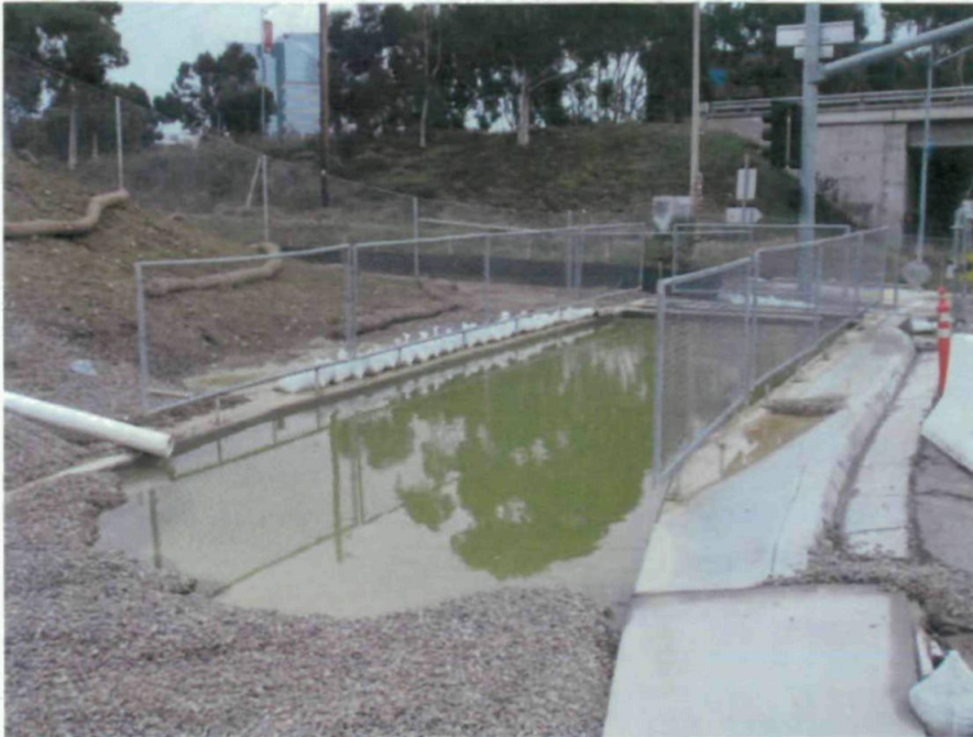
View of settling basin. Appears to be functioning but nearing capacity. More rain expected.
