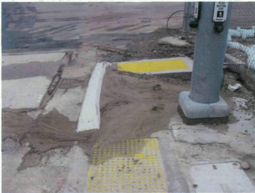
Some sediment has been captured by curb, but is nearing height of the curb.
