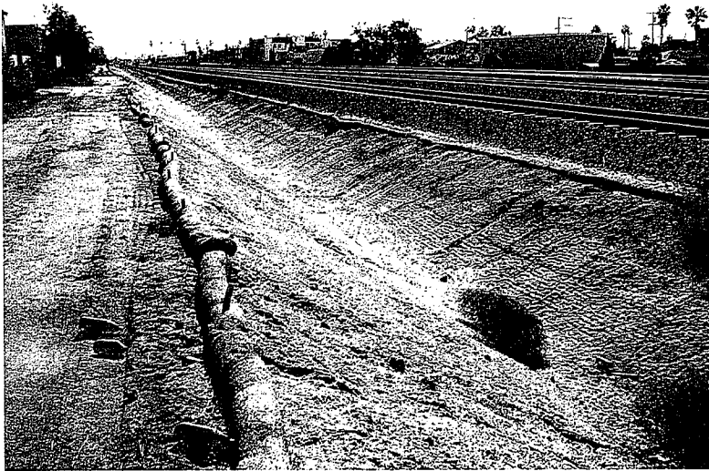
5. A long expanse of the channel is unstabilized.
