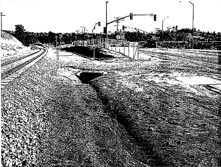
10. Earthen channel lacks stabilization.
