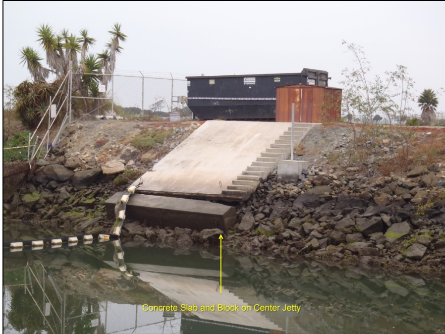
Figure 5. Concrete slab and concrete block on the center jetty towards the discharge channel (32.613648, -117.097880)
