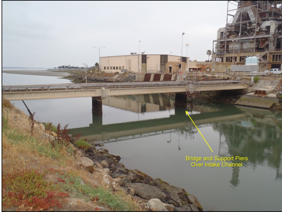
Figure 3. Bridge and support piers over the intake channel (32.613782, -117.097355) (note that the bridges and support piers over the intake and discharge channels are identical)
