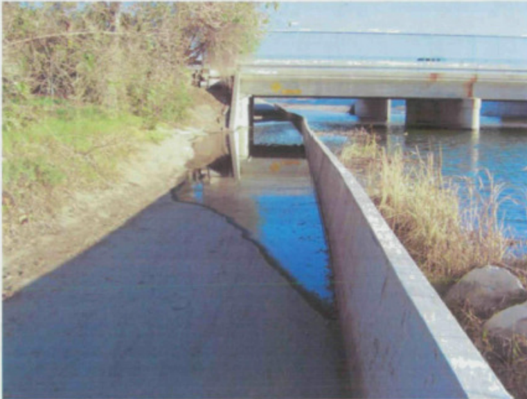
Photograph 2 San Juan Bike Trail, within the project site, looking north at PCH.
