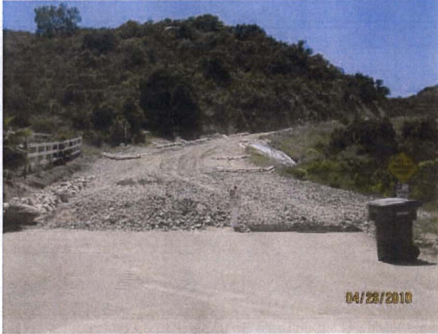
Photo 3. Stabilized Construction Entrance.
