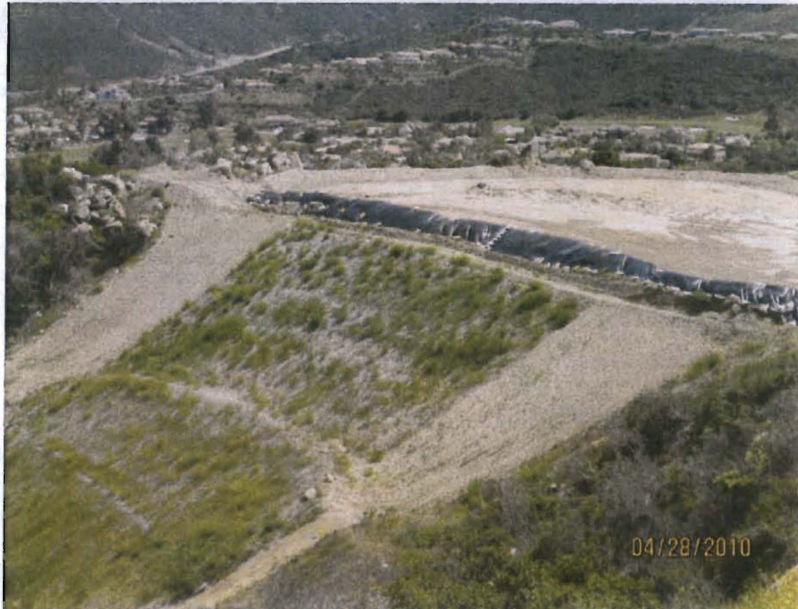
Photo 11. Graded Eitzen pad (no. 3 on the Site Map). Note temporary detention berm covered with Visqueen at edge of pad.
