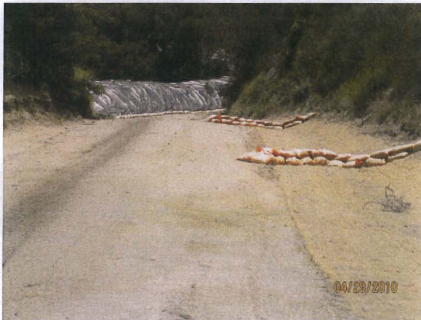
Photo 16. Looking down Cheeks Road to Lower Basin. Note erosion control mat and sandbags on inside of road
