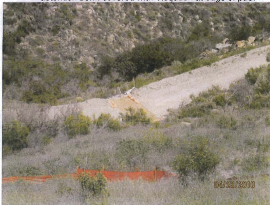
Photo 12. Eitzen driveway. Note temporary erosion control mat and Visqueen down drain BMP where swale crosses drive.
