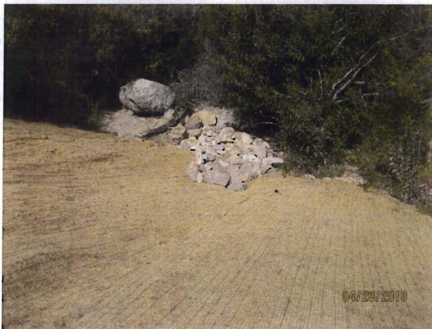
Photo 8. Looking downstream at the outlet and rip-rap below the Entrance Basin. Note jute netting on slope and undisturbed canyon below
