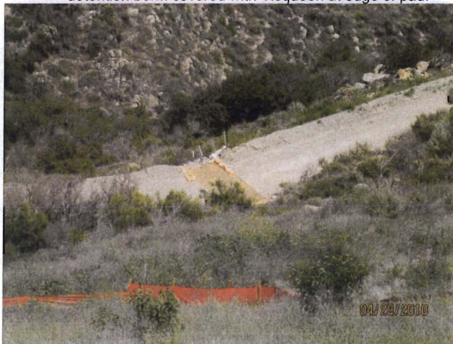
Photo 12. Eitzen driveway. Note temporary erosion control mat and Visqueen down drain BMP where swale crosses drive.
