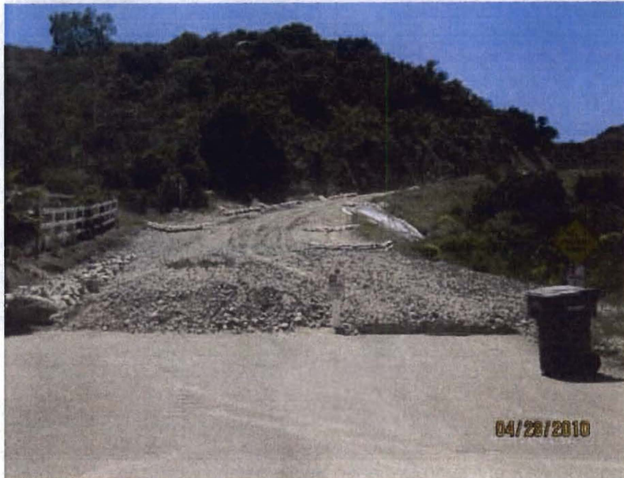
Photo 3. Stabilized Construction Entrance.
