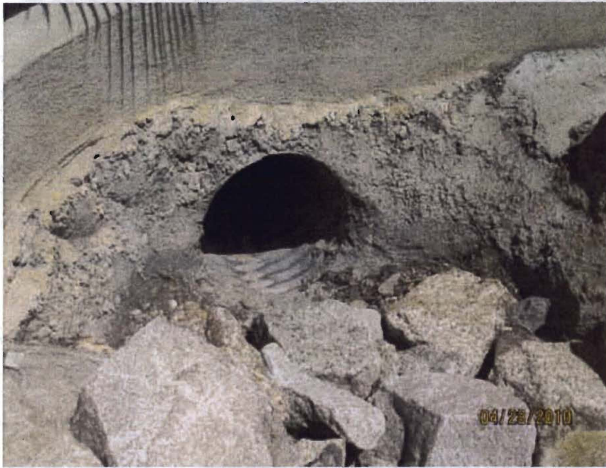
Photo 9. Culvert inlet at Claremont Street which collects Via Vista Grande run off water
