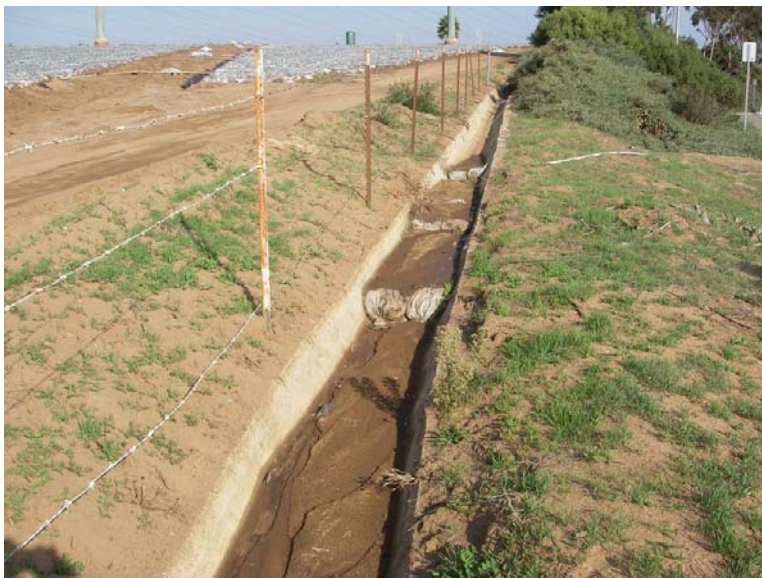
Figure D-5. Use of Sandbags near Strawberry Fields, Cannon Rd. near Interstate 5, Carlsbad Watershed.
