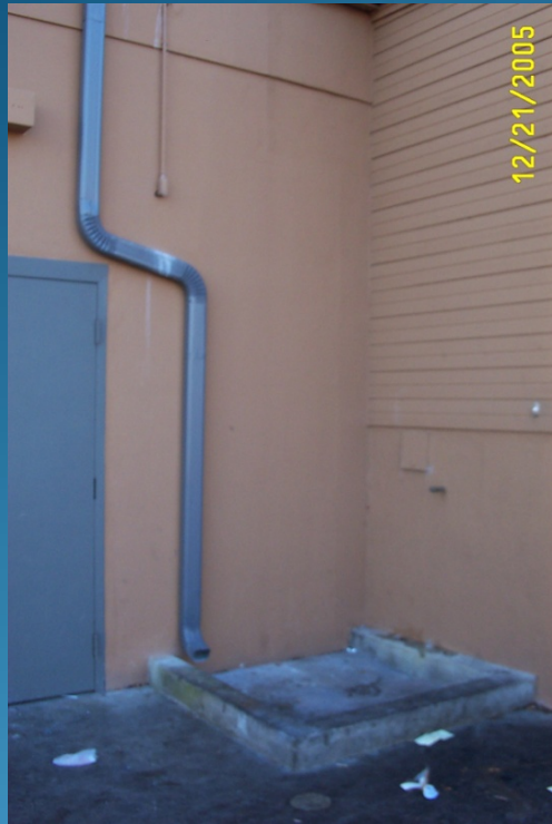
Gutter discharging to mop sink: Inflow & Infiltration
