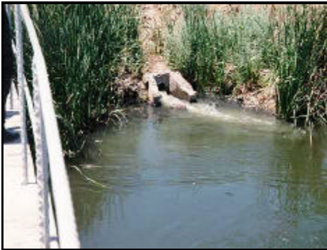
Figure 172: Raw sewage spill to New River (Jun 1995)
