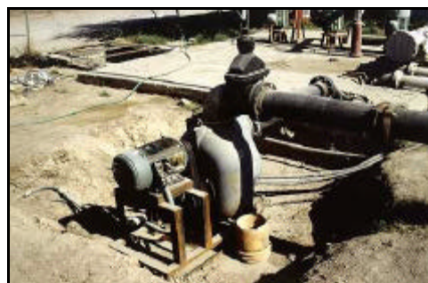
Figure 137: Gonzalez-Ortega Pumping Plant (Apr 1994)
