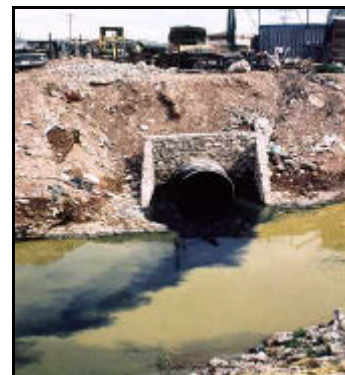
Figure 162: Raw sewage discharge from Mexicali II Collector to Mexicali Drain (Mar 1995)
