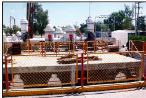
Figure 191: Pumping Plant No. 1 (Aug 1997)
