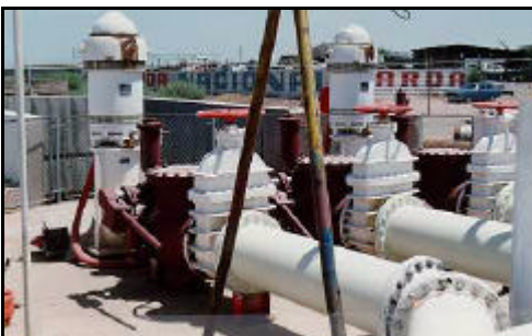
Figure 175: New check valves and manifold installed at Pumping Plant No. 1A (May 1995)
