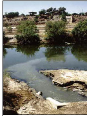
Figure 141: Bypass of raw sewage from Pumping Plant No. 1 (Aug 1994)
