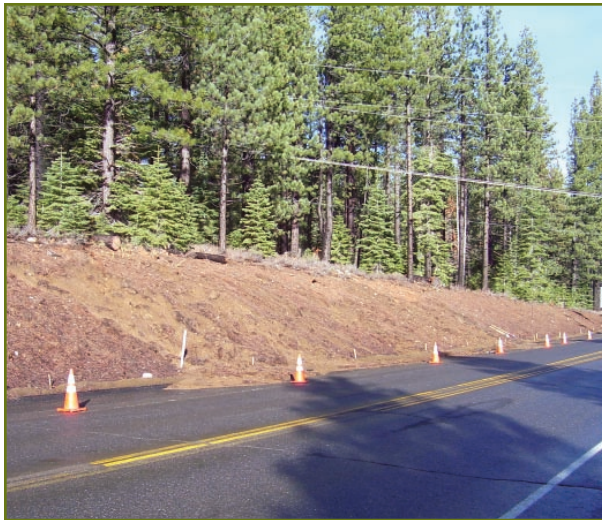
Slope failures following large storm event – December 2005.
