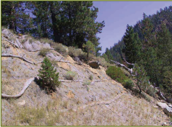
1- Project site with failing BMPs in 2002, before treatment.
