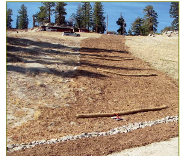
Test plots were integrated into this post-construction restoration treatment following installation of a waterline at Heavenly. The treatment area was simply divided in half and two different soil amendments were used.
