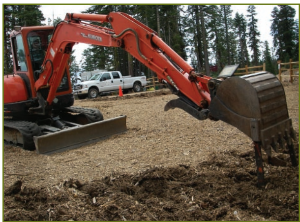
Infiltration tines mounted on excavator bucket being used to loosen soil and incorporate wood chips.
