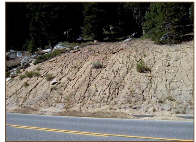
This road cut exhibits evidence of high runoff and erosion resulting from lack of infiltration capacity and vegetation.
