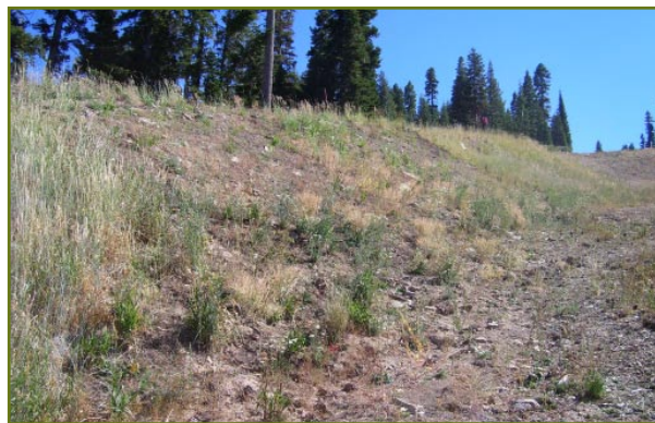
Northstar Superpipe – failure caused by over-irrigation (top); repaired slopes with proper irrigation (center); stabilized slopes two years after treatment (bottom).
