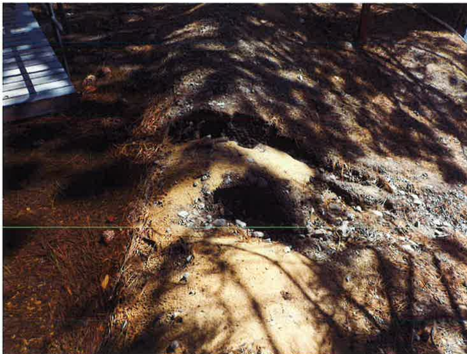
April 20, 2017. Eroded berm at STA WEST 2+40 looking east showing signs where water surface elevation in swale exceeded the design water surface elevation causing erosion.
