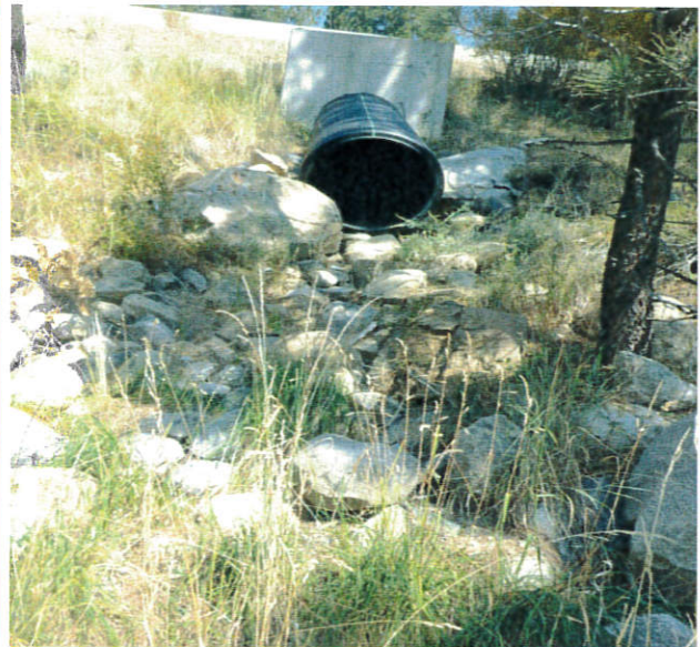
Terminus of culvert on east side of slope from east bound I 80. Good rock protection at terminus of culvert and minimal erosion issues noted, however flow from culvert likely eventually drains to channel noted in photos below.
