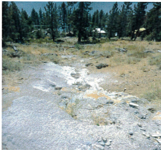
Heavy channalization from flow downslope of I80 - looking downslope @ terminus of lower TDPUD access road.
