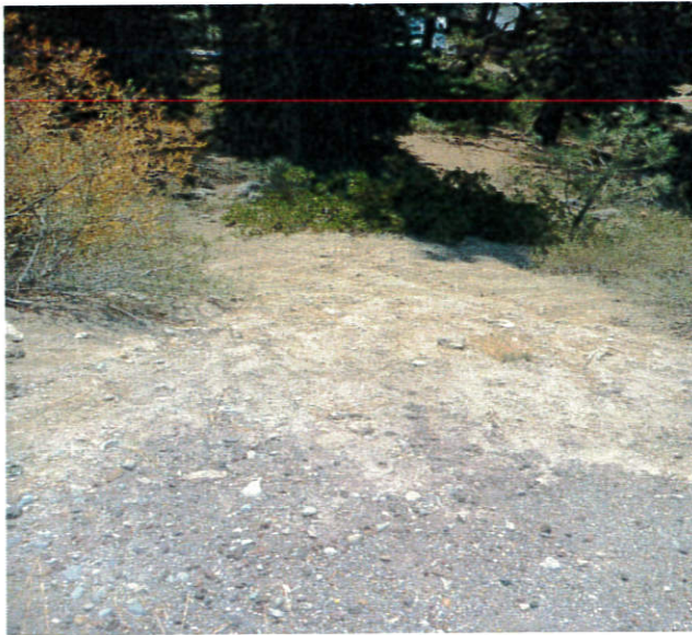
Hillslope failure & erosion just below culvert that is conveying water flow from natural seep/spring across of Donner Lake Road. No infrastructure in place to direct stormwater flow and minimize erosion.
