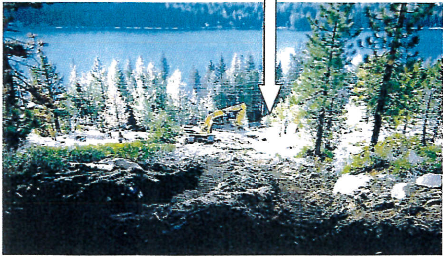
Photo 23. The TDPUD installed a water pipeline from the Cedar Point alignment downslope to West Reed Avenue in 2004. Photo taken August 2004.
