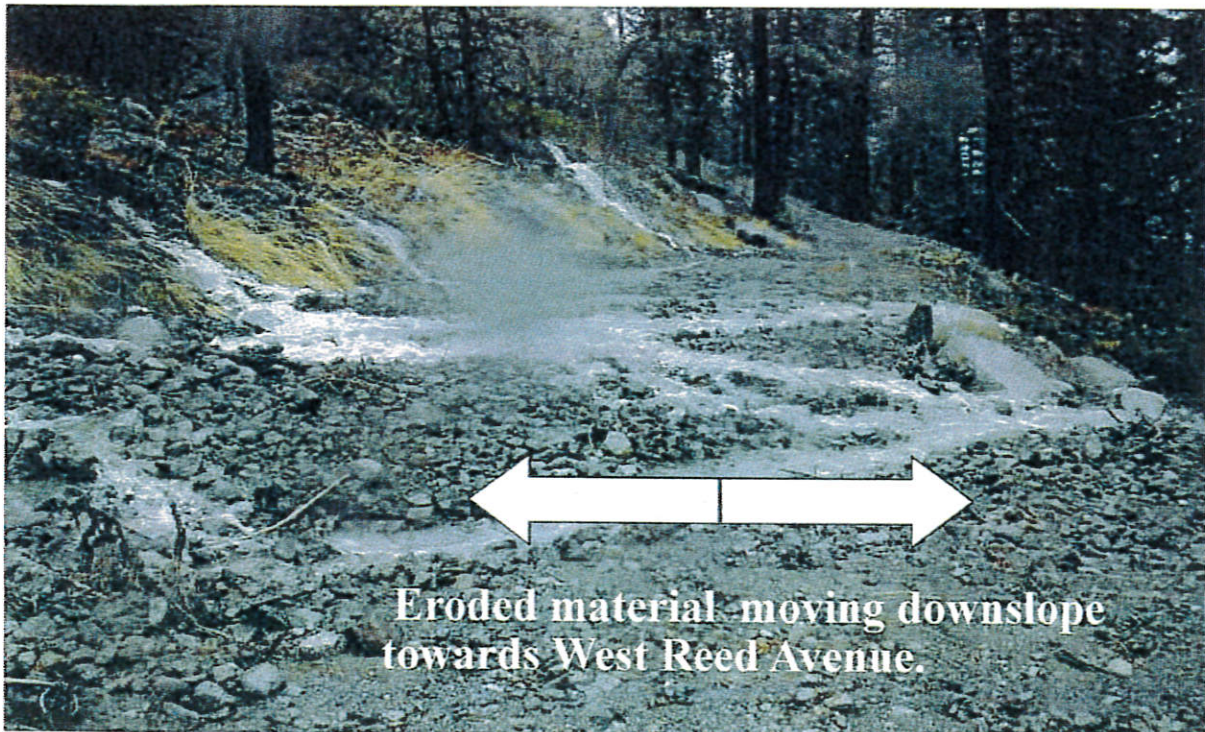
Photos 3 and 4. High velocity runoff outside Caltrans culvert and eroded material being transported downslope. Photo taken December 31, 2005.
