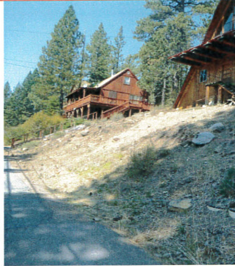
Denuded hillslope on private property residence looking west along West Reed Avenue - unprotected hillslope and lack of stormwater drainage ditches likely to contribute excess sedimentation to public and private properties downslope including Donner Lake.
