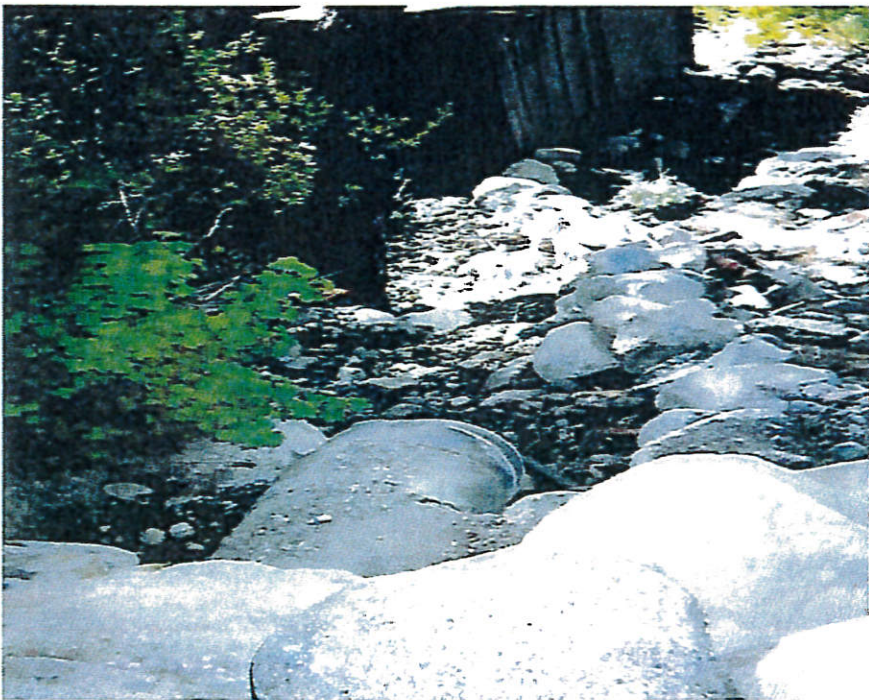
Photo 10. A culvert outfall on the south side of West Reed Avenue does not convey runoff effectively as debris clogs the inlet on the north side of the road. Photo taken May 29, 2006.
