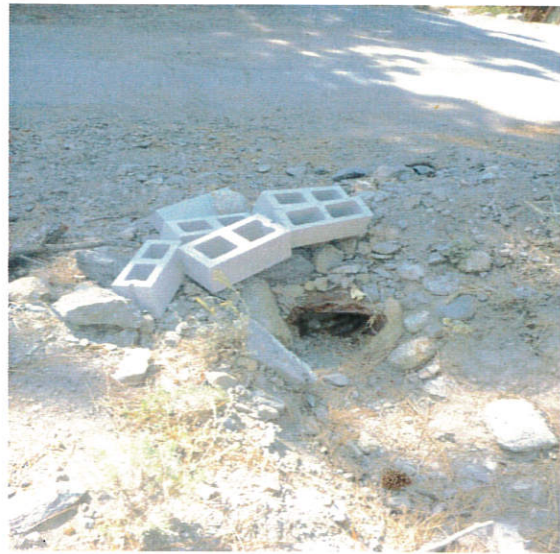
Deteriorated, undersized and unmaintained culvert crossing West Reed Avenue – inlet for flow from channel located below I 80 in photos 1-4 above.
