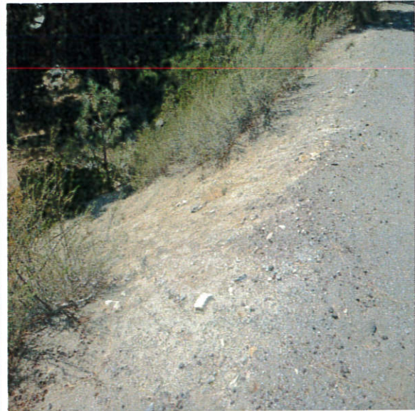
Looking downslope in area in previous photo: below culvert that is conveying water flow from natural seep/spring across of Donner Lake Road. No infrastructure in place to direct stormwater flow and minimize erosion.
