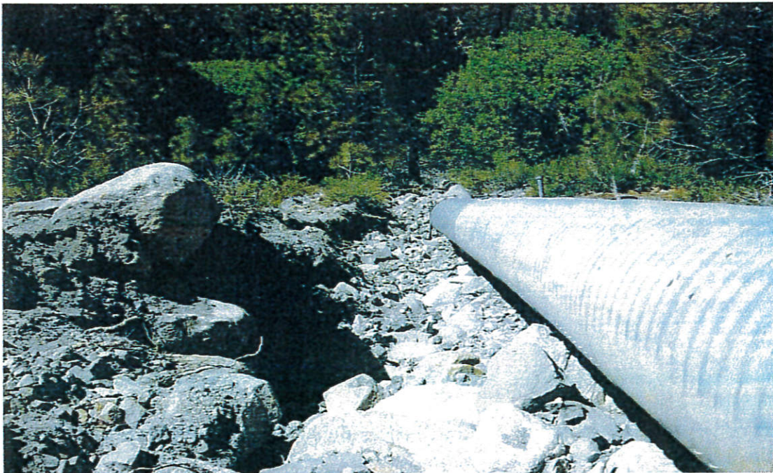
Photo 2. Looking downslope along the culvert where eroded material is being transported down the hillside above West Reed Avenue. Photo taken June 6, 2006.
