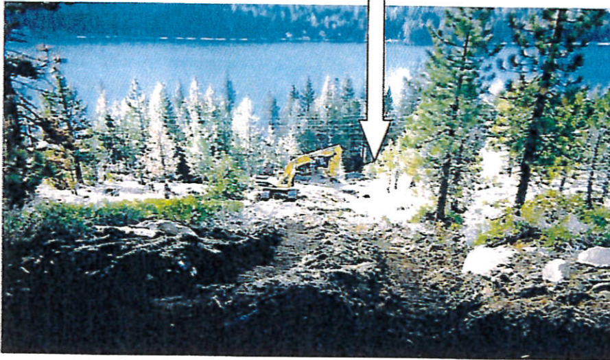
Photo 23. The TDPUD installed a water pipeline from the Cedar Point alignment downslope to West Reed Avenue in 2004. Photo taken August 2004.
