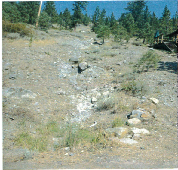
Increased channelization and incision downslope of I-80. Looking upslope from location of undersized culvert located on West Reed Avenue.
