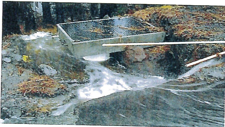
Photo 13. Eroded water utilities on West Reed Avenue.
