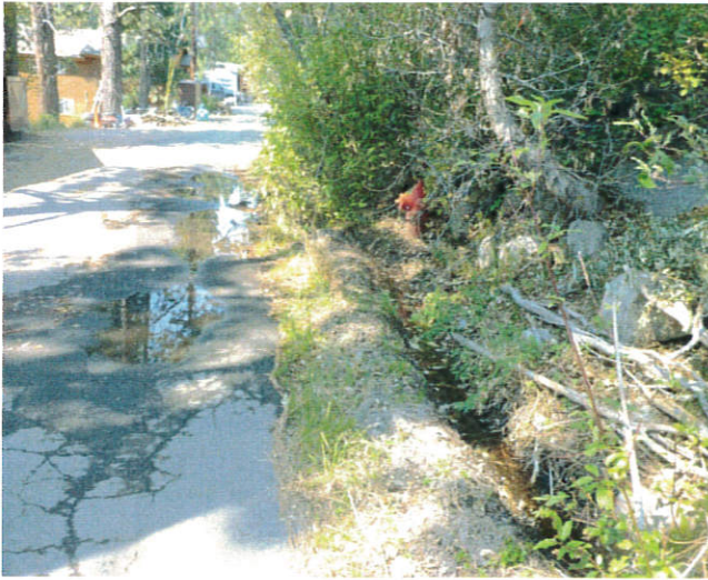
Natural seep below 15014 West Reed Avenue – no infrastructure in place to direct stormwater flow resulting in overtopping and flooding of roadway.
