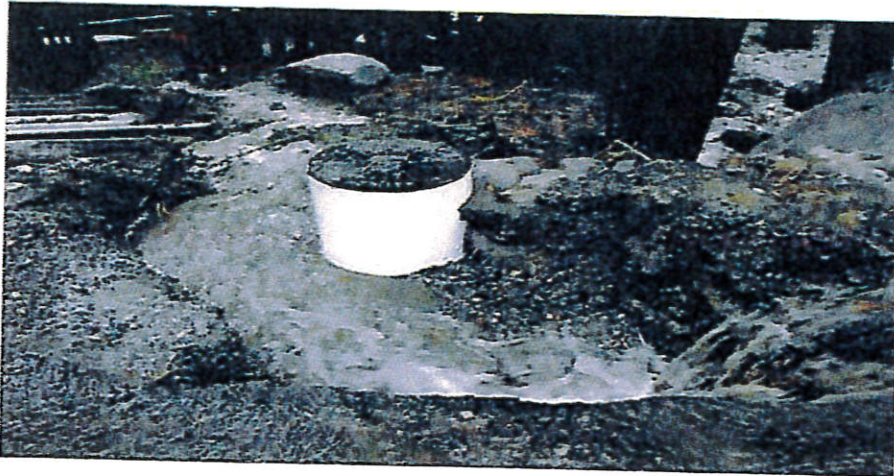
Photo 11. Eroded water utilities on West Reed Avenue.
