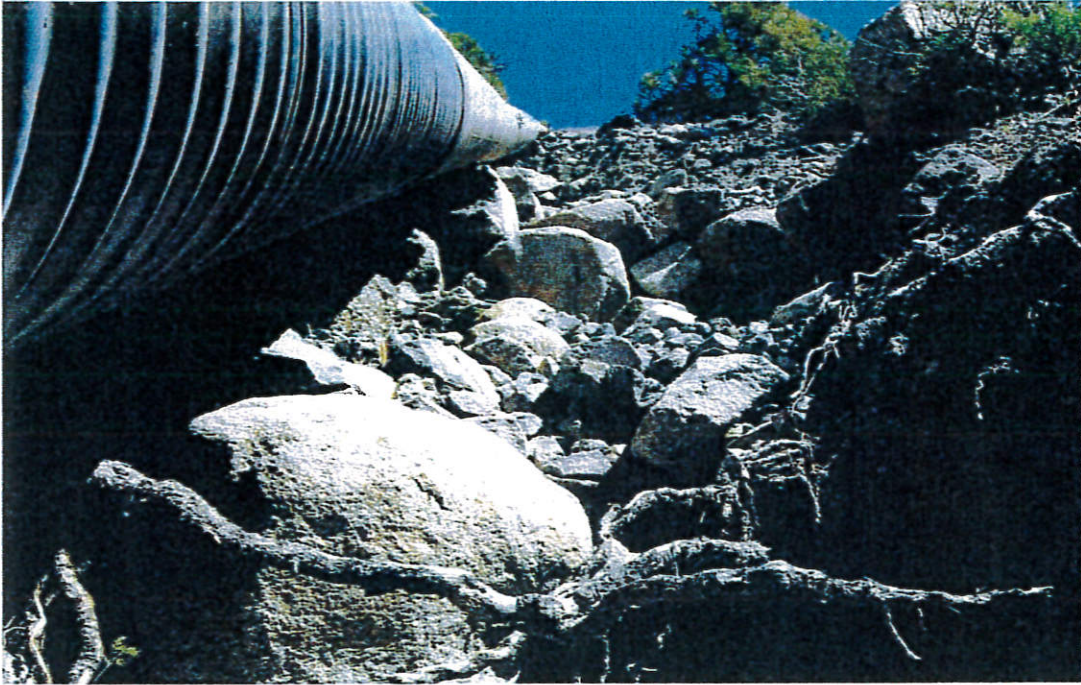
Photo 1. Looking upslope along at the Caltrans culvert on the east end of the hillside above West Reed Avenue. Photo taken June 6, 2006.
