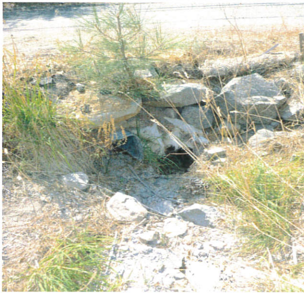
Deteriorated, undersized and unmaintained culvert crossing West Reed Avenue - potential for flooding & compromising of utility lines
