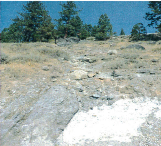
Channalization across bedrock material from I80 - top third of slope – looking uphill.
